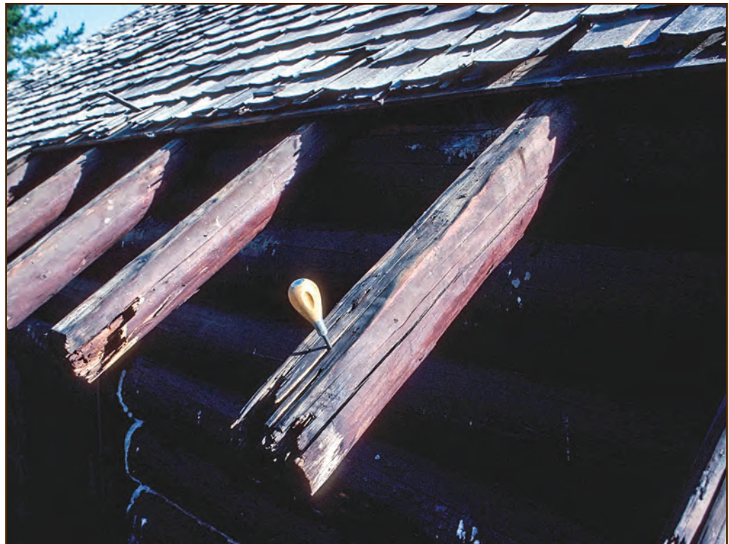
Figure 48—The awl stuck into this rafter tail shows how deeply the rot has penetrated. Rot is very common on rafter tails like these that extend beyond the edge of the roof.
