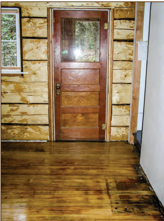
Figure 310—The refinished kitchen floor of the Adams Ranger’s House shows evidence of past heat damage from a wood stove that someone didn’t properly shield. Because it shows no evidence of heat damage, it’s easy to tell that someone previously replaced a short floorboard where the stove once sat.
