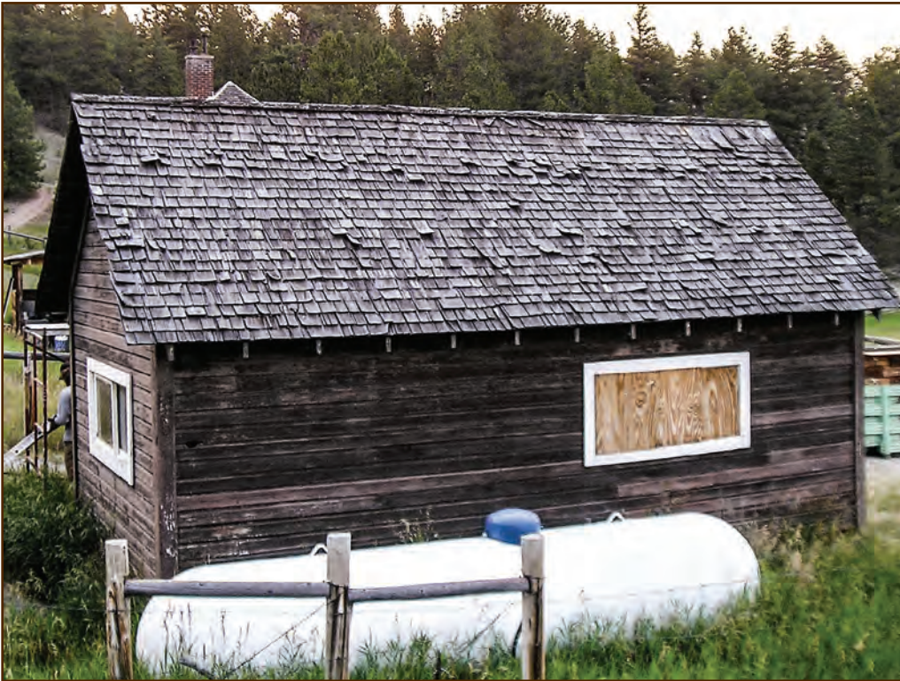
Figure 234—More than 20 percent of the shingles on this roof are worn out or damaged, so you should replace the roofing.
