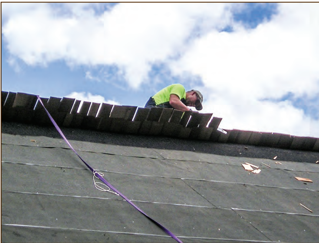
Figure 274—This roofer is using a small hand saw to trim the ends of the cock's comb ridge for the replacement roofing on the Moose Creek Wilderness Station Office/Cookhouse building (Nez Perce National Forest, Northern Region). Although the roof that the preservation crew replaced had a shingle ridge cap, historic photos showed that the original ridge cap was a cock's comb. The crew took the opportunity presented by the need for new roofing to restore the original configuration.
