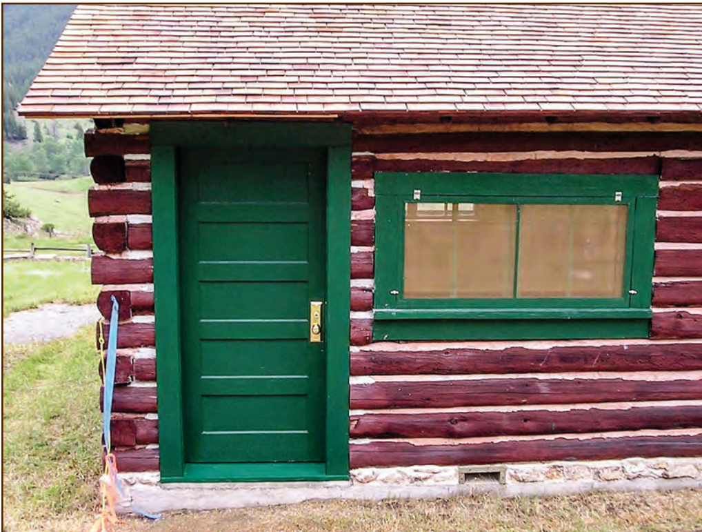
Figure 305—As part of the renovation of the 1905 House at the Main Boulder Station (Gallatin National Forest, Northern Region), preservation crewmembers constructed a new door to meet accessibility requirements. The crew installed the door on the back of the cabin; it has the same number and configuration of panels as the historic doors, but is 36 inches wide. The crew later constructed a stoop to provide level access from the yard to the door.
