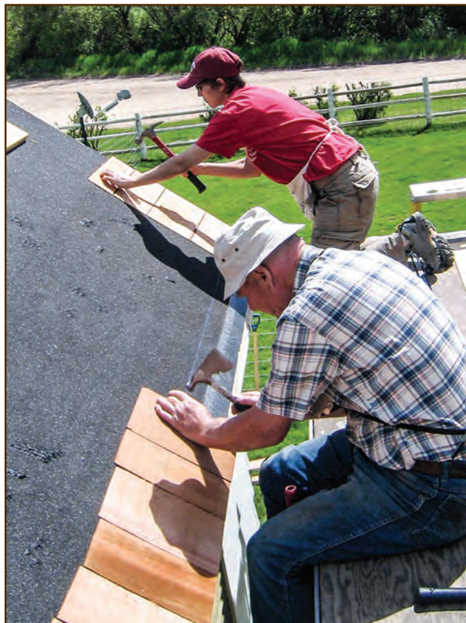
Figure 239—The roofer at the top of the photo is laying raker shingles. The other roofer is laying the starter course. Before laying any shingles, the crew covered the entire roof with ice and water shield underlayment.
