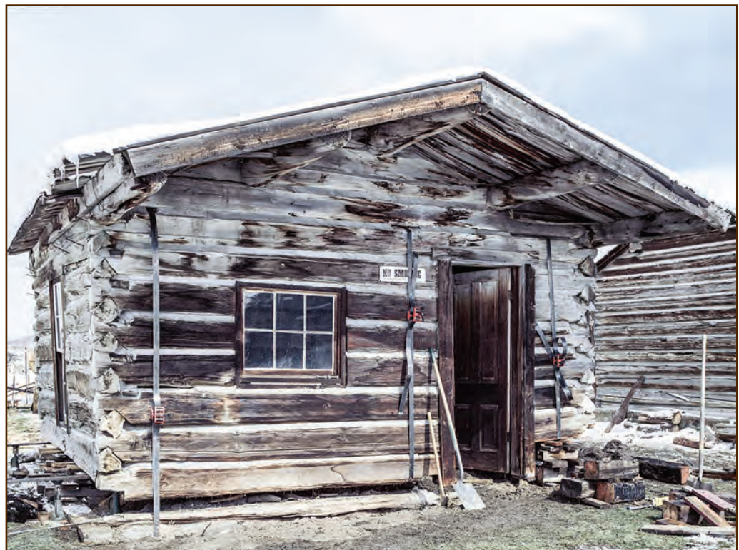
Figure 64—Preservation carpenters used band clamps to hold the logs together on the front of this cabin in Nevada City, MT, during a renovation project. Clamping allowed the carpenters to remove the rotten sill logs and to raise the building without risking collapse.
