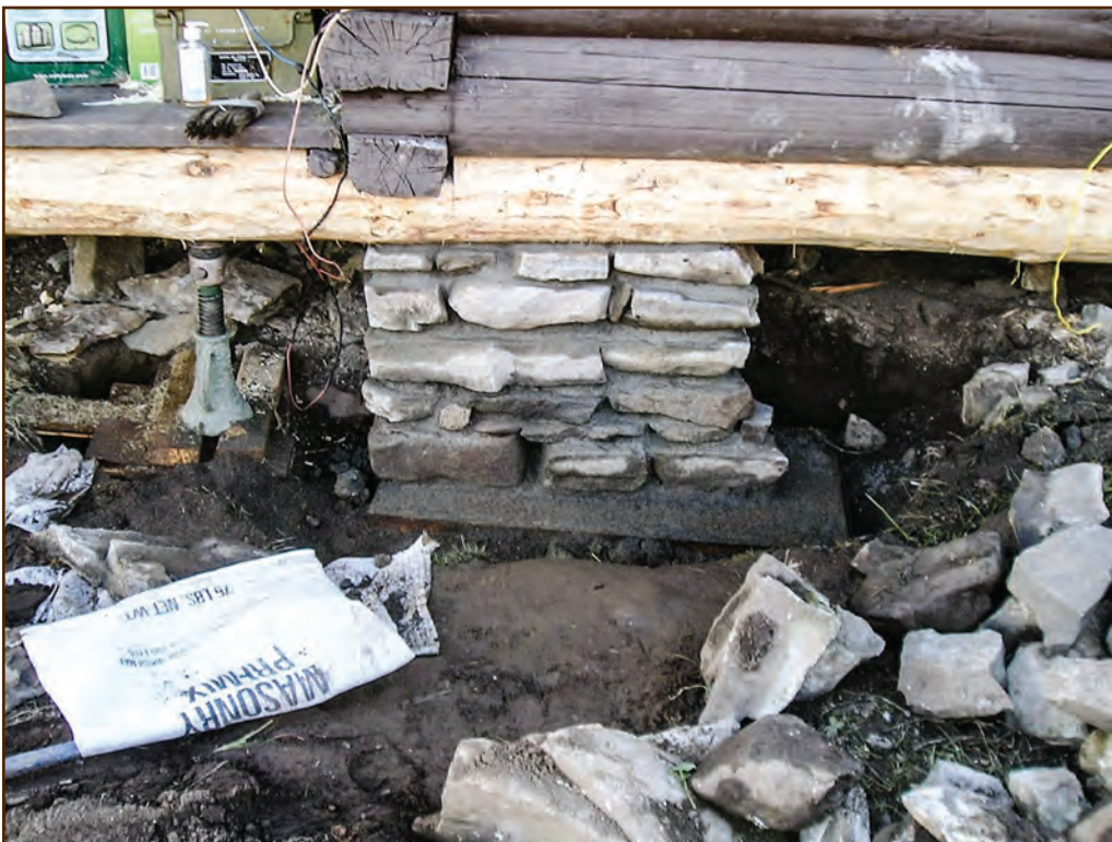
Figure 82—A preservation crewmember constructed a new footing and sturdy flat stone pier at the Badger Cabin within the Lewis and Clark National Forest, Northern Region.
