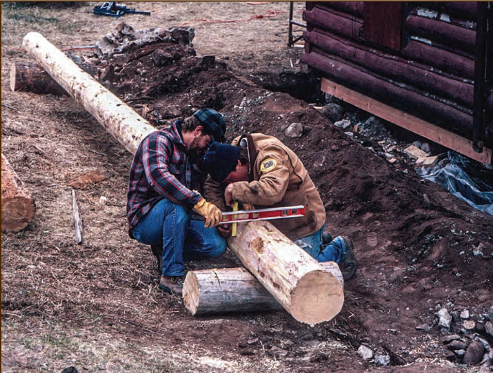
Figure 152—To make shaping a replacement log easier, place it next to the cabin in its correct orientation. Measure to ensure that the dimensions closely match those of the log that you removed.
