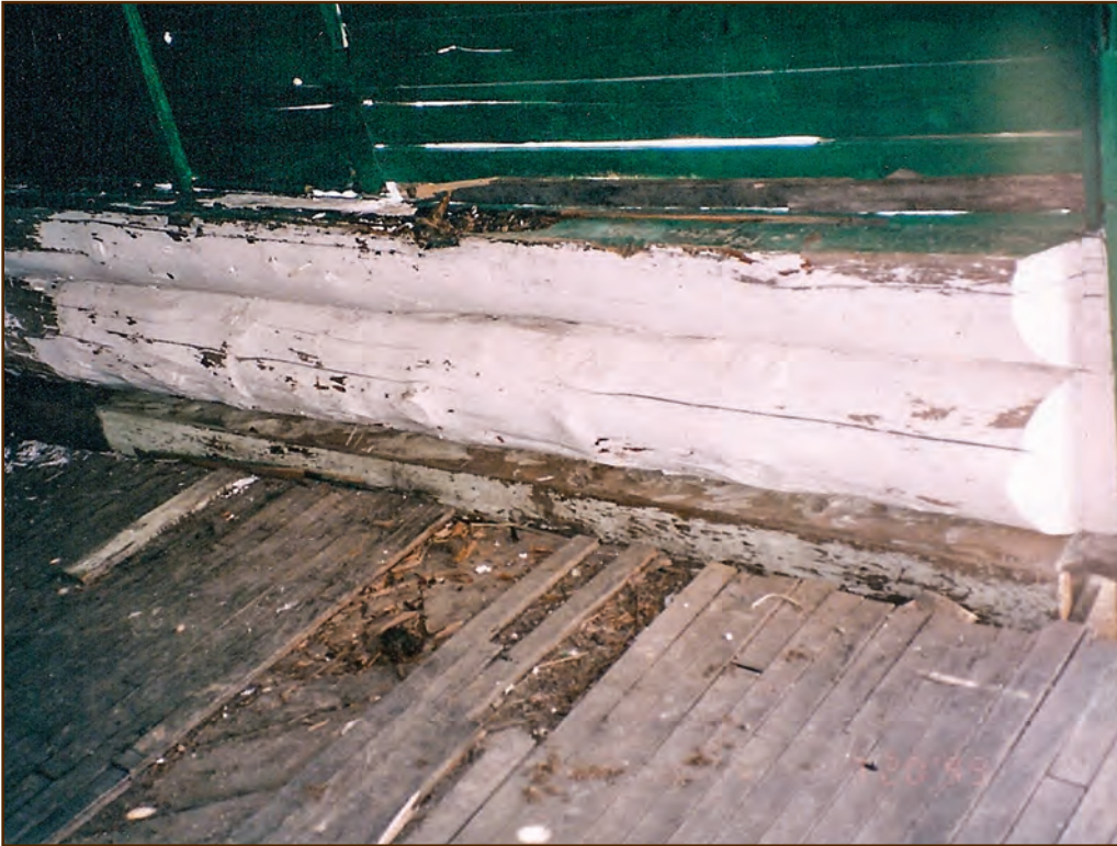
Figure 311—The flooring inside the Square Mountain Lookout (Salmon River Ranger District, Nez Perce National Forest, Northern Region) was deteriorated beyond repair and preservation crewmembers had to completely remove it.
