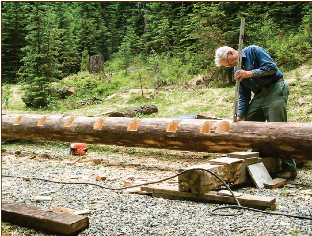
Figure 129—Preservation crewmembers prepared this new sill log for the Adams Ranger’s House (Salmon River Ranger District, Nez Perce National Forest, Northern Region) using the deteriorated original sill log (not shown in the photo) as a pattern for the floor joist notching.
