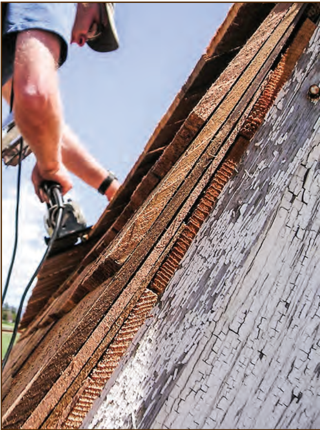
Figure 261—This edge view of the stud barn roof at the Nine Mile Ranger Station (Lolo National Forest, Northern Region) shows rakers and three layers of shingles. The shingles immediately above the fascia are rakers. You can tell which shingles are rakers because their end grain is exposed, rather than the edge grain exposed on the sides of other shingles.
