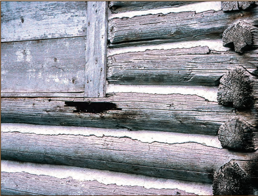
Figure 166—This whitewashed cabin has a small, deteriorated area beneath one of the windows.
