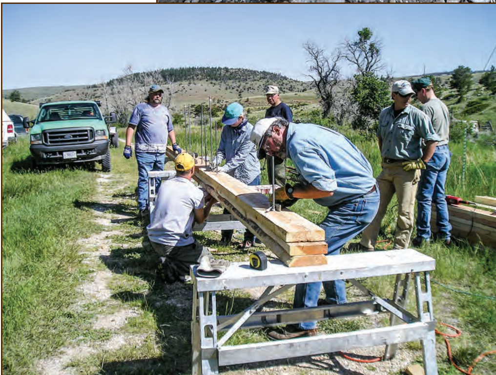
Figure 70—This preservation crew is constructing needles to support the Sage Creek Cabin (Custer National Forest, Northern Region) while they raise and replace the sill and spandrel logs.
