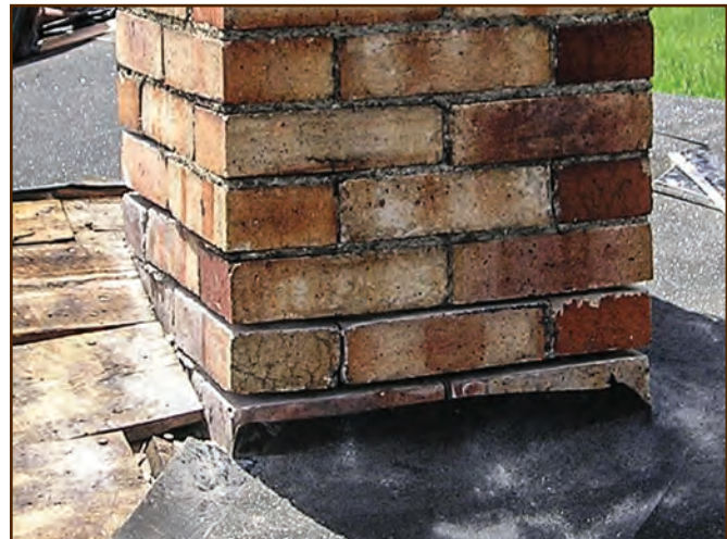
Figure 242—In preparation for reflashing, a preservation crewmember raked out the mortar from the joints on the chimney of the house at the Main Boulder Station (Gallatin National Forest, Northern Region) built in 1905.
