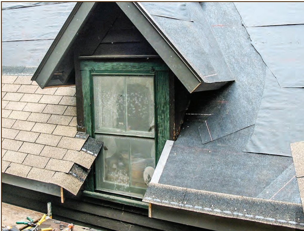
Figure 284—As shown in the lower right of this photo, roofers created an asphalt shingle starter course for the roof of this historic log cabin by cutting the tabs off regular shingles. Note the position of the adhesive spots near the eave edge of the shingles. The original builders constructed the log part of the cabin, known as “the Homestead,” in the early 1800s on what is now the Bradford District (Allegheny National Forest, Eastern Region). The owner added frame wings in the early 1900s.
