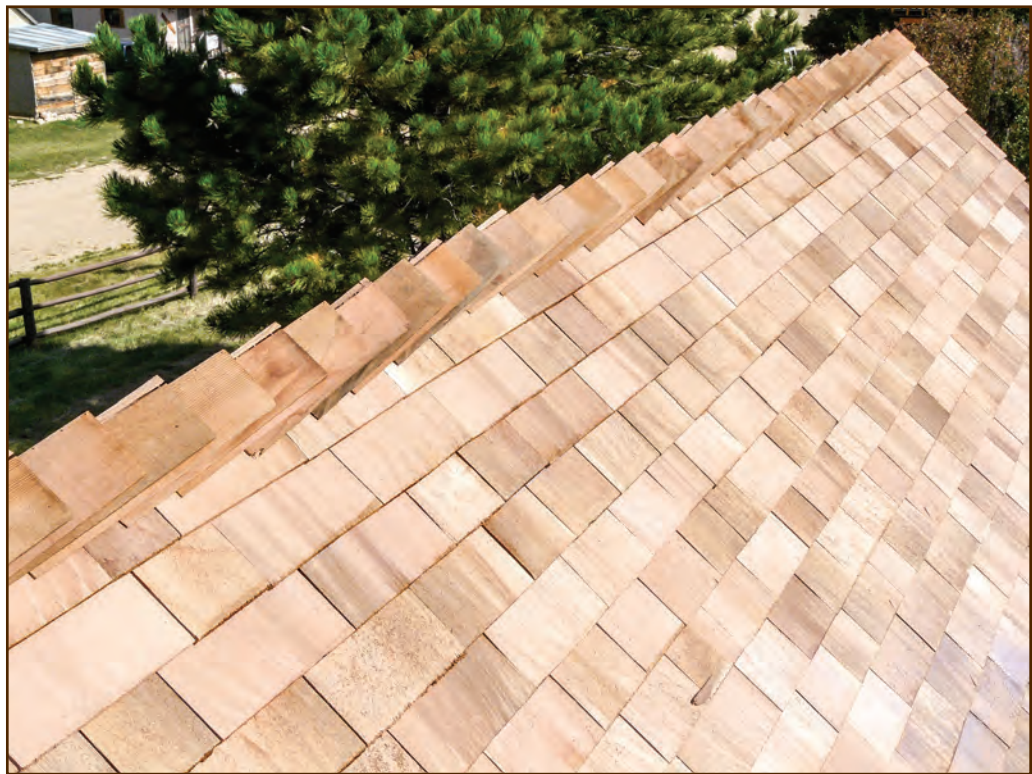
Figure 275—Preservation crewmembers constructed this shingle ridge cap when they replaced the roofing at the Ninemile Ranger Station (Lolo National Forest, Northern Region).
