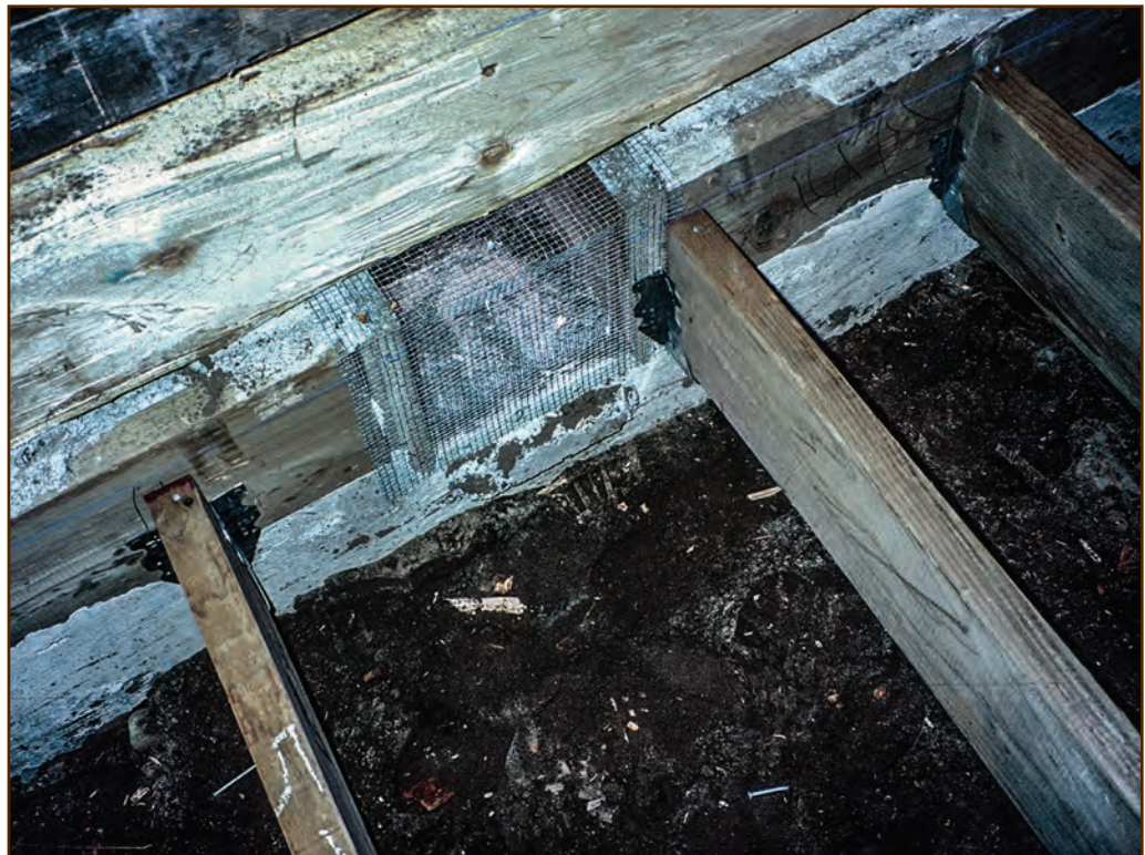
Figure 134—Preservation crewmembers replaced the failed original floor joists in one of the early 20th-century cabins at the OTO Ranch in the Gallatin National Forest, Northern Region. They used dimensioned lumber joists supported by steel joist hangers that they attached to treated lumber rim joists set into the new concrete foundation.
