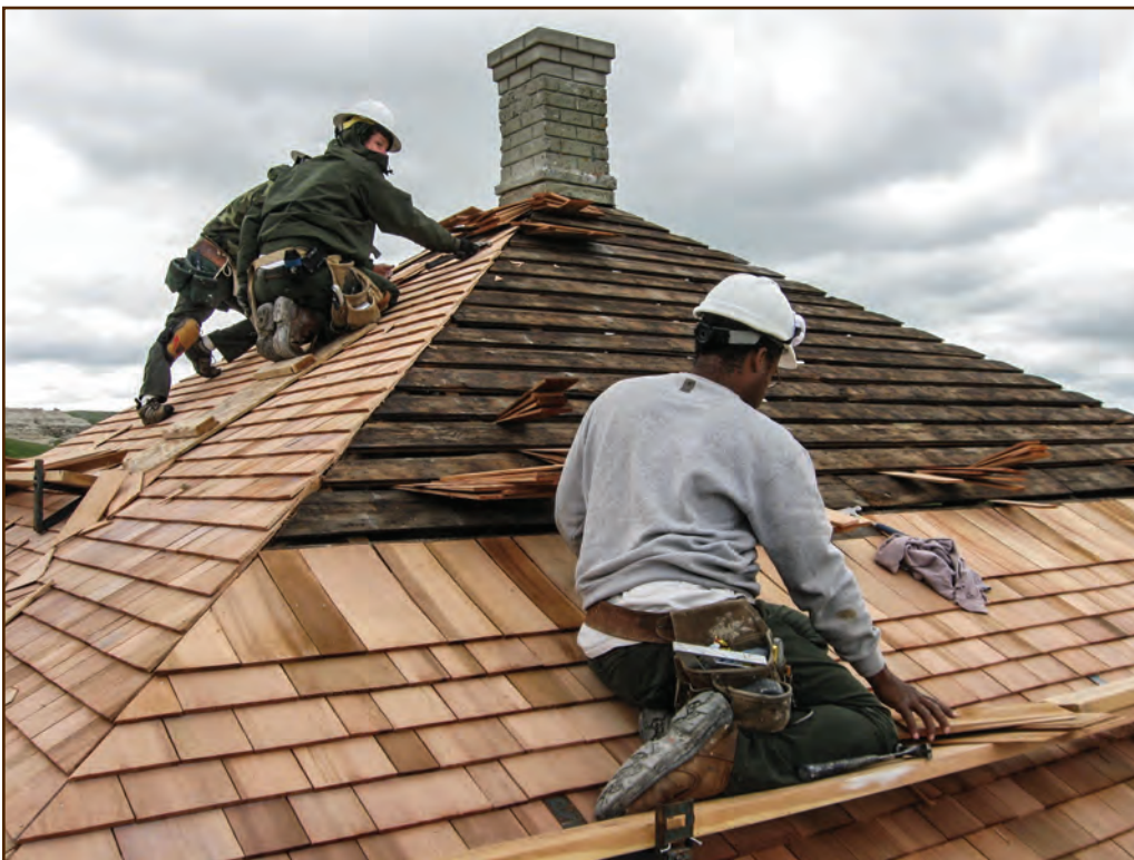
Figure 50—Roofing replacement often is the first renovation chore on a log cabin. These National Park Service preservation workers are replacing the shingle roof on the Jessie Elliott Ranger Station of the Custer National Forest. It's not a log building—it's the only stone ranger station in the Northern Region. The builders constructed it around 1913 and installed wood shingles in the same manner as on log buildings of the same vintage. Full scaffolding with railings all around the roof provided fall protection on this project.
