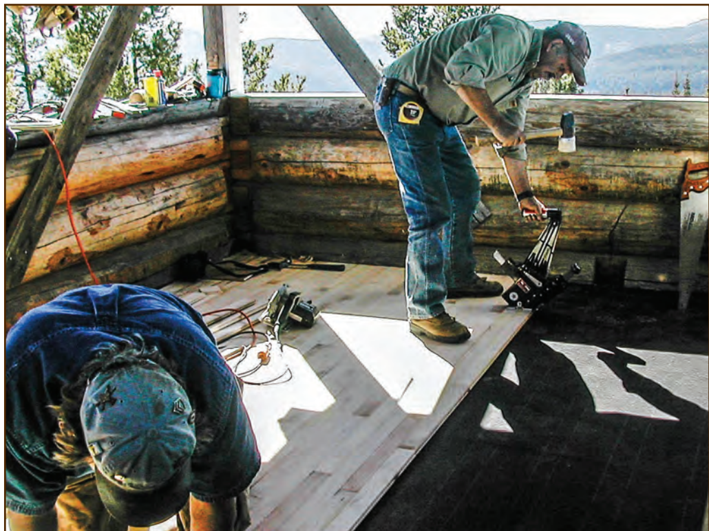
Figure 312—After the Northern Region Historic Preservation Team repaired or replaced deteriorated logs, floor joists, and subflooring at the Square Mountain Lookout, they installed new flooring of the same type as the original.
