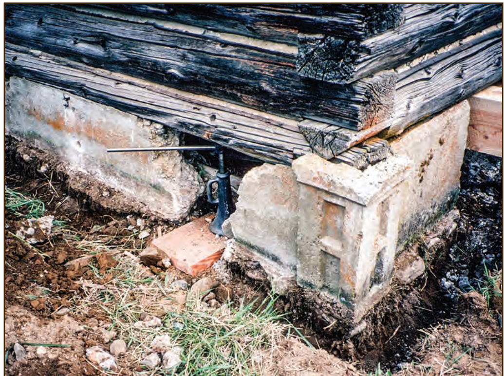
Figure 84—Preservation crewmembers removed part of the foundation to allow placement of a jack (center) and a timber needle (far right) to support the cabin during foundation removal and log replacement. The crewmembers replaced these temporary supports with steel needles on cribbing before forming the new foundation.
