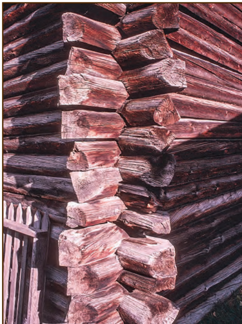
Figure E17—Irregular, wedge-shaped crown ends that extend beyond the corner notches.
