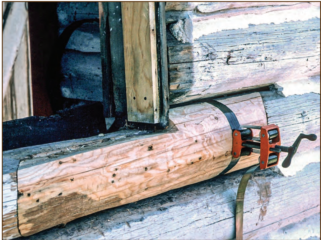
Figure 171—The preservation carpenter removed the original windowsill and cut the top of the splice down for the windowsill. He applied epoxy adhesive behind the patch and secured the splice to the original wall with a band clamp. The splice fit perfectly into the notch. Next, he drilled the dowel holes.
