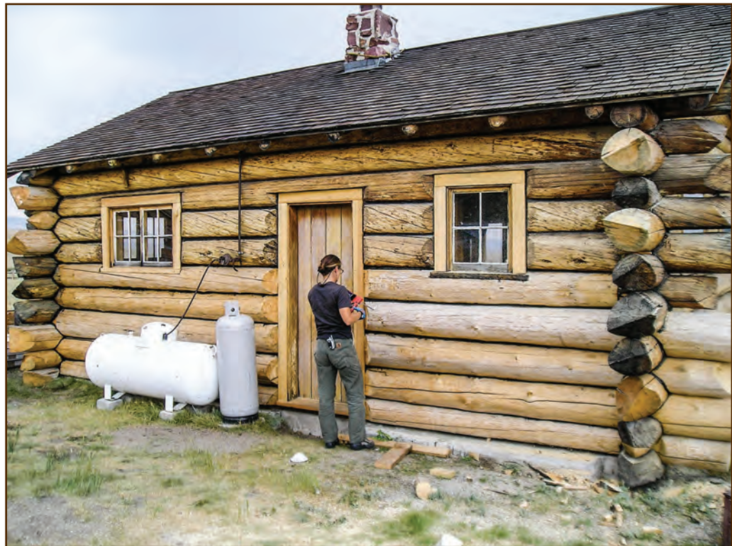
Figure 194—This worker is using a caulking gun to apply tar daubing between the logs of the Horse Prairie Cabin (Beaverhead-Deerlodge National Forest, Northern Region).
