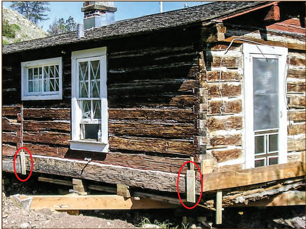
Figure 62—Preservation carpenters attached markerboards (circled) made from 1-inch-thick lumber to the sill logs of the Sage Creek Cabin (Custer National Forest, Northern Region) so they could use a transit to check that the building rose evenly and remained level.
