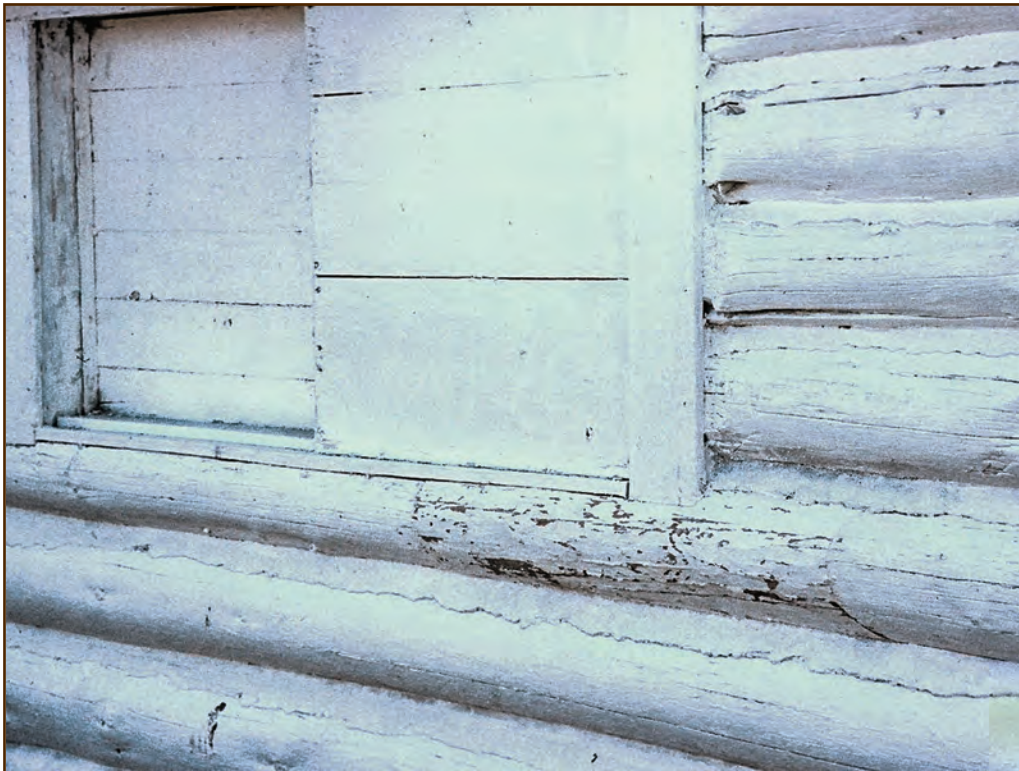
Figure 173—The preservation carpenter has repaired the chinking and daubing and applied whitewash to the patch, which is just barely noticeable. The whitewash didn't penetrate the new splice as well as the original logs. By the time the cabin needs another application of whitewash, the splice will have weathered and will absorb the whitewash more uniformly.
