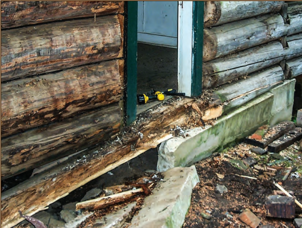
Figure 39—A diverted stream that overflowed and reclaimed its original streambed undermined the foundation of the Adams Ranger's House (Salmon River Ranger District, Nez Perce National Forest, Northern Region). Because the building wasn't in use and funding was unavailable, no one repaired the foundation damage for about 40 years. During that time, the lack of foundation support led to damage to sill logs and other parts of the cabin.
