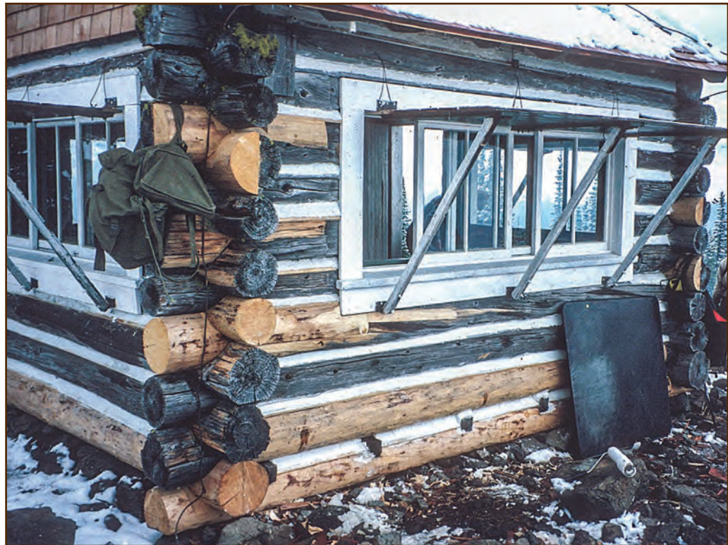
Figure 131—Preservation crewmembers replaced or repaired several logs of this lookout cabin. Just as in the original structure, the crewmembers set the floor joists in notches cut into the top of the sill logs. These notches are visible from the outside of the lookout cabin.
