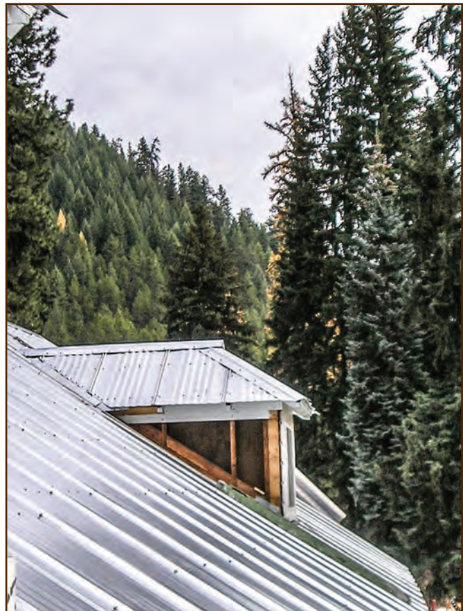
Figure 281—The ridge cap is the final element that you install on a metal roof. In this photo, the roof is complete, but the preservation crew has not yet replaced the siding on the dormer.
