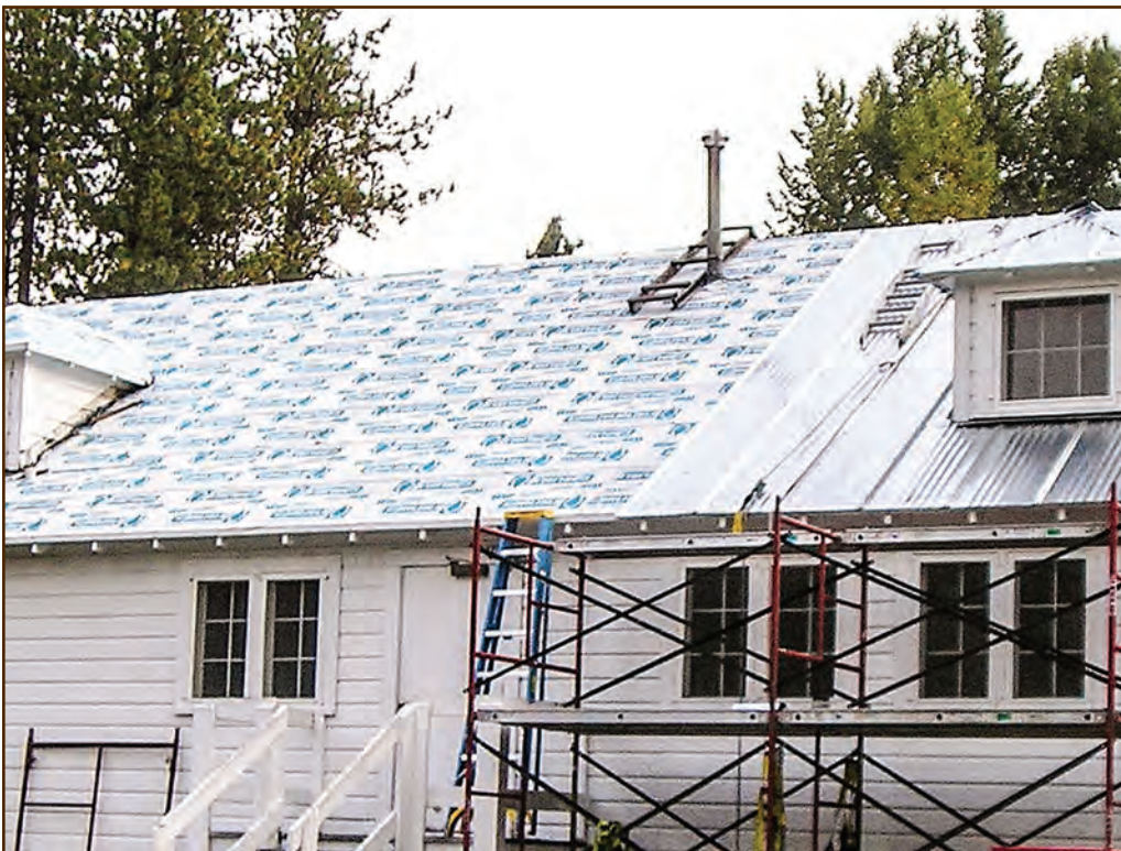
Figure 278—Preservation crewmembers are laying a new corrugated metal roof over ice and water shield on the Sav-enac Tree Nursery Bunkhouse (Lolo National Forest, Northern Region), built in 1930. The roof is the same kind you would find on log cabins of a similar vintage that have metal roofs.
