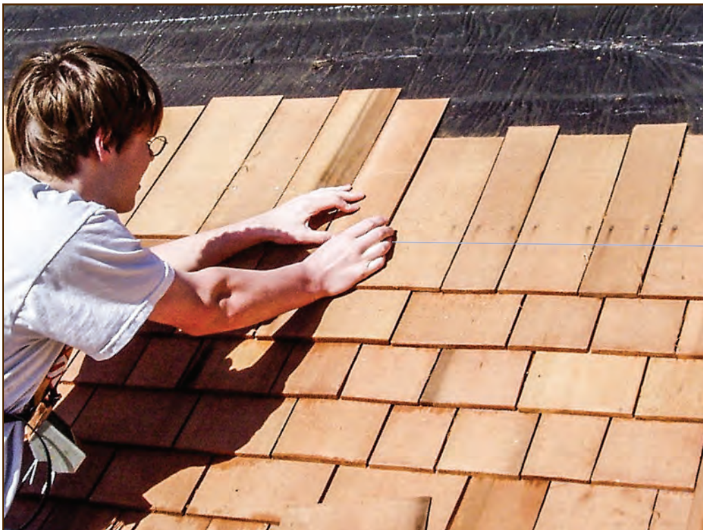
Figure 266—This roofer is laying shingles in courses on the west house at the historic Ninemile Ranger Station (Lolo National Forest, Northern Region). The shingle courses are evenly spaced due to careful measuring and the use of chalklines. The chalkline for the current course is visible in the photo. The horizontal spaces between the shingles are reasonably even.
