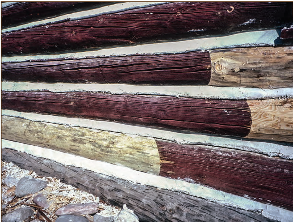
Figure 165—This photo shows several trimmed Dutchman splices on exterior logs of the Judith Guard Station (Lewis and Clark National Forest, Northern Region). Although the species and diameter of all patches match well, the middle splice does not match the original log grain pattern as well as the top and bottom splices do.
