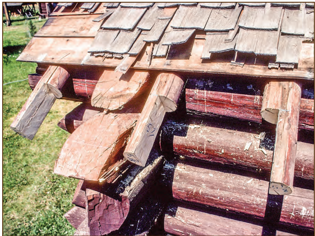
Figure 189—Preservation crewmembers cut these rafter tails to the same pattern to make shaping and attaching the replacement rafter tails easier. They oriented the joints with a vertical splice cut to maximize the strength of the joint and to allow any water that might enter the joint to drain.
