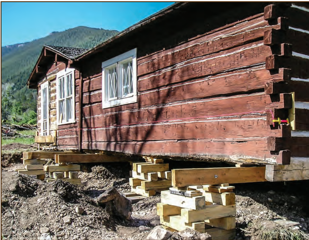
Figure 76—Preservation carpenters raised the Sage Creek Cabin (Custer National Forest, Northern Region) 18 inches during a 2-week period, using needles, jacks, and cribbing.
