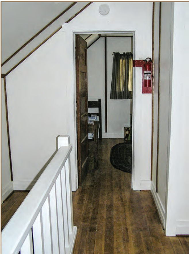
Figure 316—Preservation crewmembers repaired the original fiberboard panels and wood battens covering the upstairs walls of the Adams Ranger's House when they could save them and replaced the panels and battens when they couldn't.
