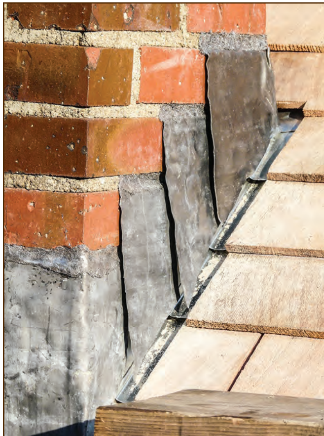
Figure 246—This closeup view of the chimney constructed in 1905 at the Zortman Guard Station within the Bureau of Land Management's HiLine District in Montana shows how the builder used lead sheets to counter flash the chimney. The builder stuffed lead wool into the masonry joints to match the original method of holding the counter flashing in place. The step flashing under the counter flashing is just barely visible.
