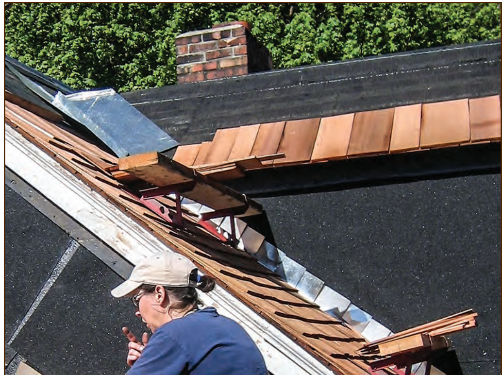
Figure 241—This roofer is installing galvanized steel step flashing and valley flashing during the reroofing of this complex roof at the historic Ninemile Ranger Station (Lolo National Forest, Northern Region).
