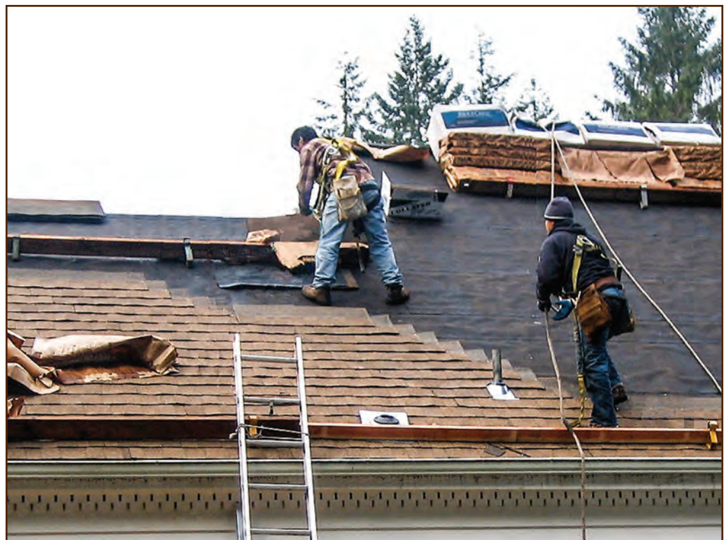
Figure 285—When the roofers replaced the roof on this 1936 residence, they applied asphalt shingles in a stair step pattern. Roofing nails are visible near the right edge of each tier of shingles. The building, located just north of Lincoln City, OR, is part of the Pacific Northwest Research Station's Cascade Head Experimental Forest.
