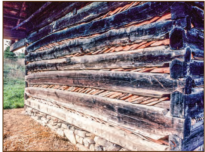
Figure E30—The builders used slate as chinking between the logs on this cabin. They laid the pieces of slate on wood blocking to angle them toward the outside of the building to help shed rain.
