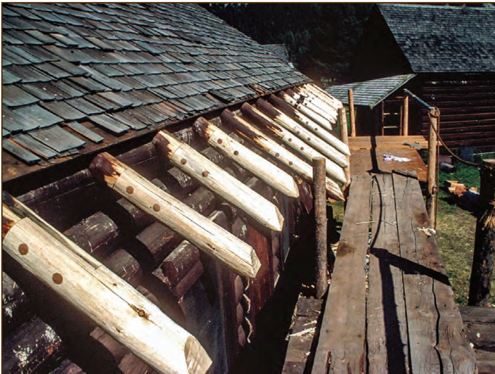
Figure 191—Preservation crewmembers replaced all the rafter tails on this building. The crew trimmed the dowels flush with the rafter tails, but the dowels still are clearly visible as darker spots. Next, the crew will stain the rafter tails using the same product as the original rafter tails. Finally, they will install new sheathing and roofing.
