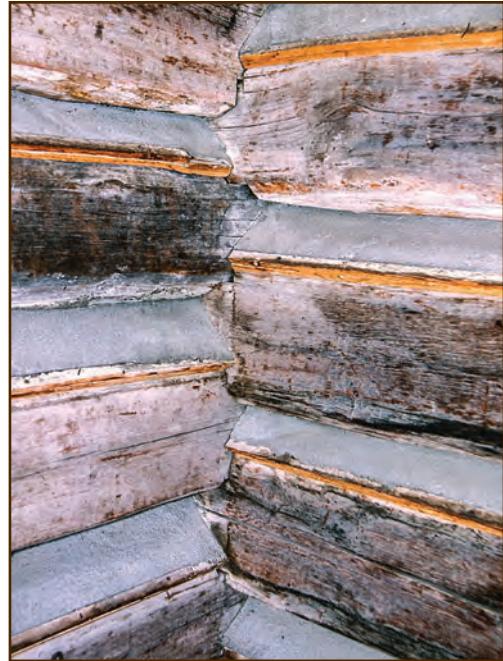
Figure E34—The builders used small pieces of wood trim as edging for the sloped daubing on this hewn log cabin. Preservation crewmembers replaced some of the edging (brighter colored wood) when they repaired the daubing.
