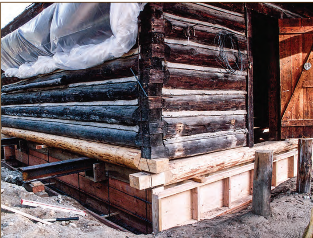
Figure 85—Preservation crewmembers replaced deteriorated logs and constructed forming for the new foundation around the steel beam needles that support this cabin.
