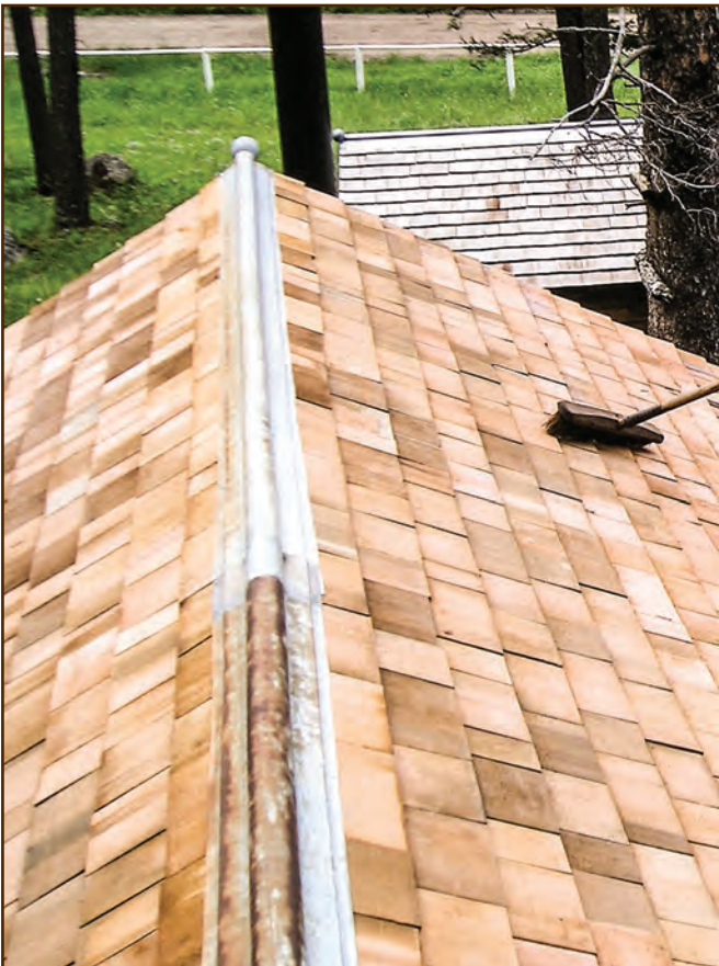
Figure 272—Preservation crewmembers carefully removed and reinstalled the original metal ridge cap after replacing the shingles on the Moose Creek Garage (Helena National Forest, Northern Region).
