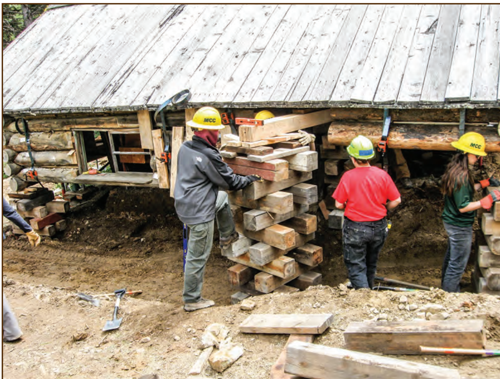
Figure 73—This crew at Garnet Ghost Town within the Bureau of Land Management's Garnet Resource Area in Western Montana employed safe cribbing and jacking techniques. They constructed a level, stable base in a crosshatch pattern to support the jacks and cribbing, then stacked the cribbing in a crosshatch pattern.
