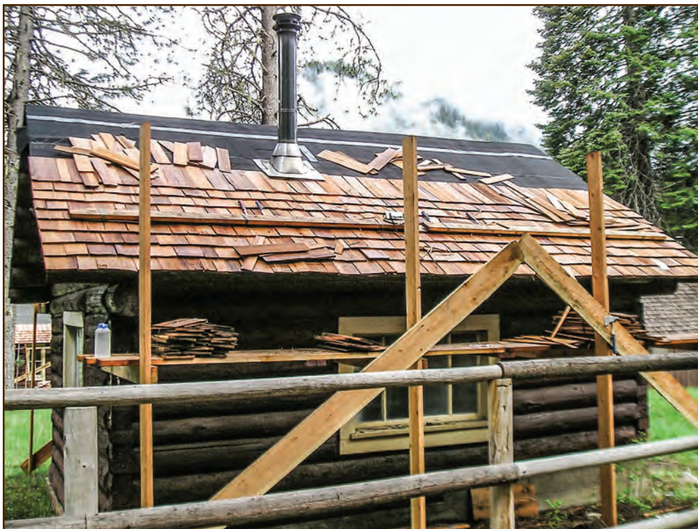
Figure 268—Roofers are installing a new shake roof on the Wash House at the Moose Creek Wilderness Station (Nez Perce National Forest, Northern Region). This 1937 log building has solid roof sheathing.
