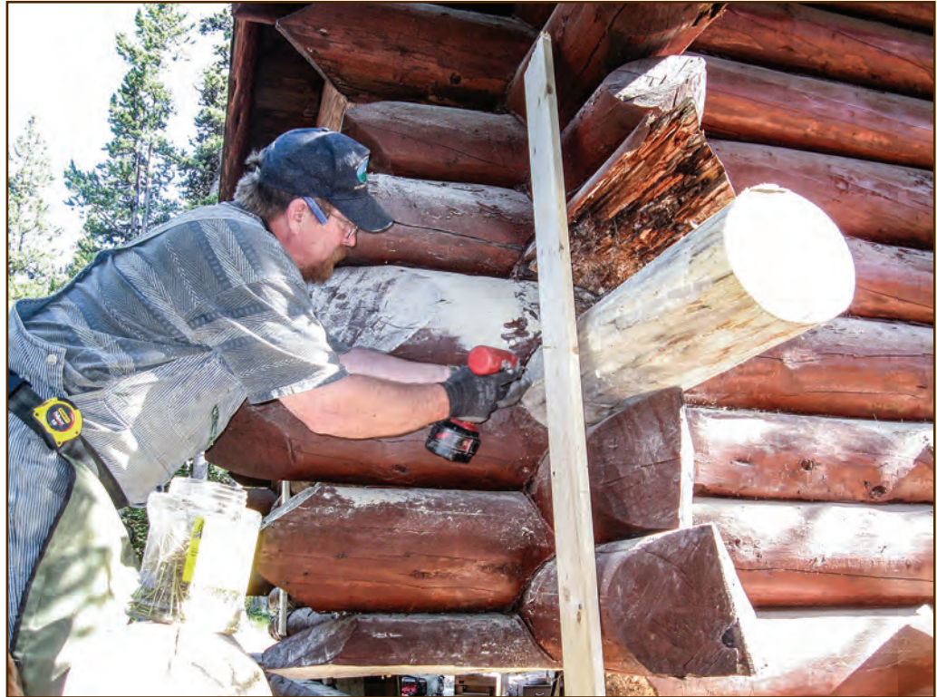
Figure 184—Kirby Matthew, now retired from the Forest Service Northern Region Historic Preservation Team, drives one of two temporary screws. He’s using the screws, a tie board, and epoxy adhesive to hold the replacement crown end in place while he drills holes for the permanent dowel connection.
