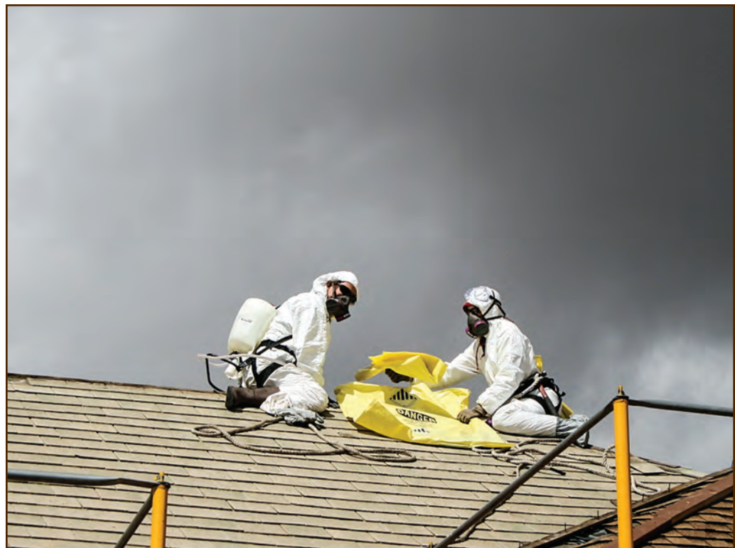
Figure 52—This properly attired and certified crew is removing asbestos shingles from a Forest Service building roof in Gunnison, CO. The asbestos shingles were under a newer layer of composition shingles.
