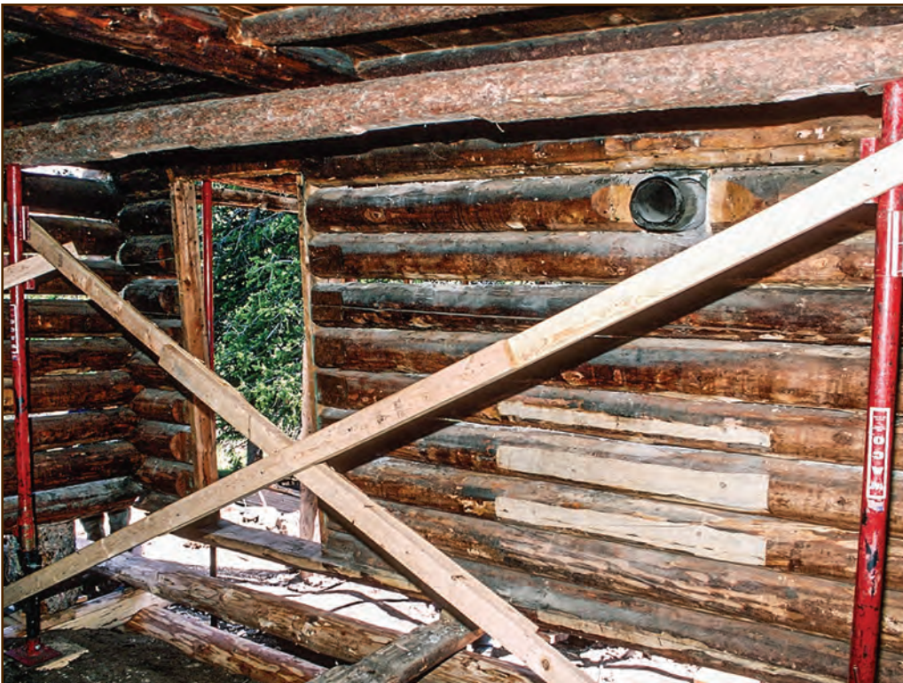
Figure 66—The roof of this cabin is temporarily supported by a beam on “X” braced shore posts.
