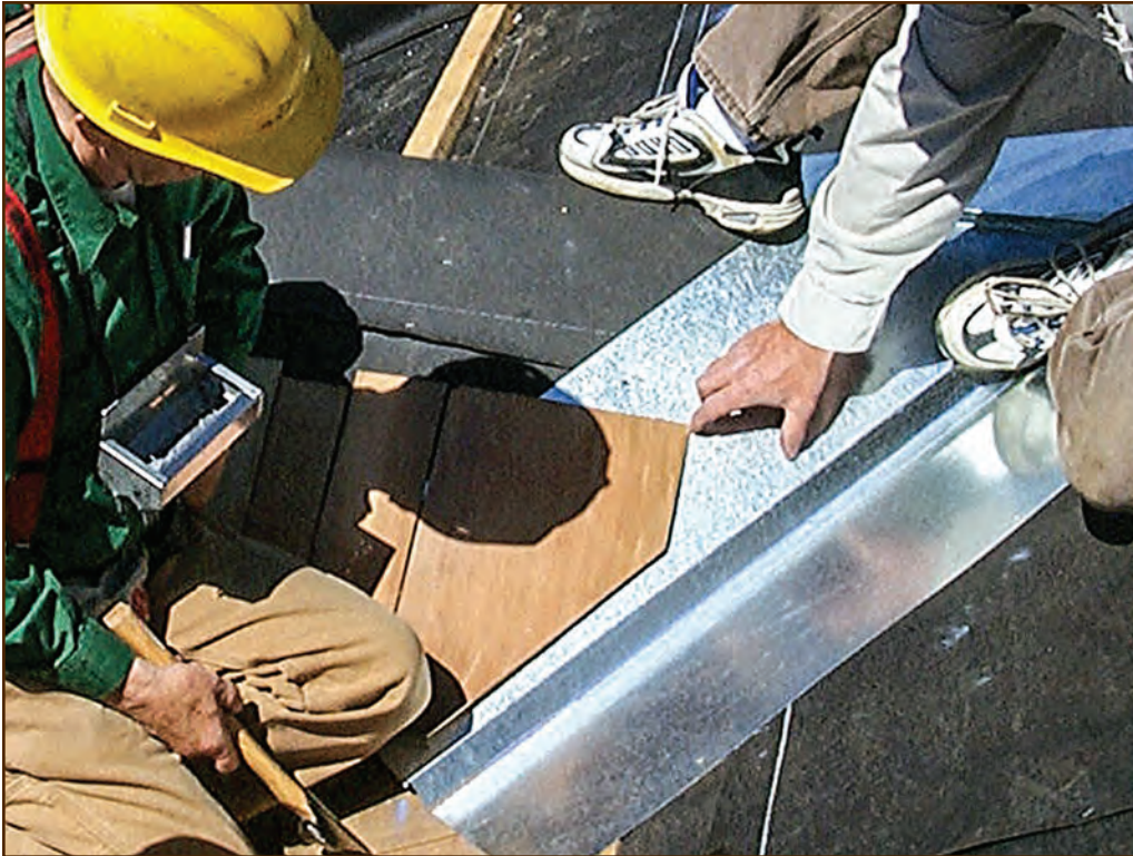
Figure 255— Preservation crewmembers used W-shaped valley flashing when they replaced the roof on this building at the Ninemile Ranger Station (Lolo National Forest, Northern Region).
