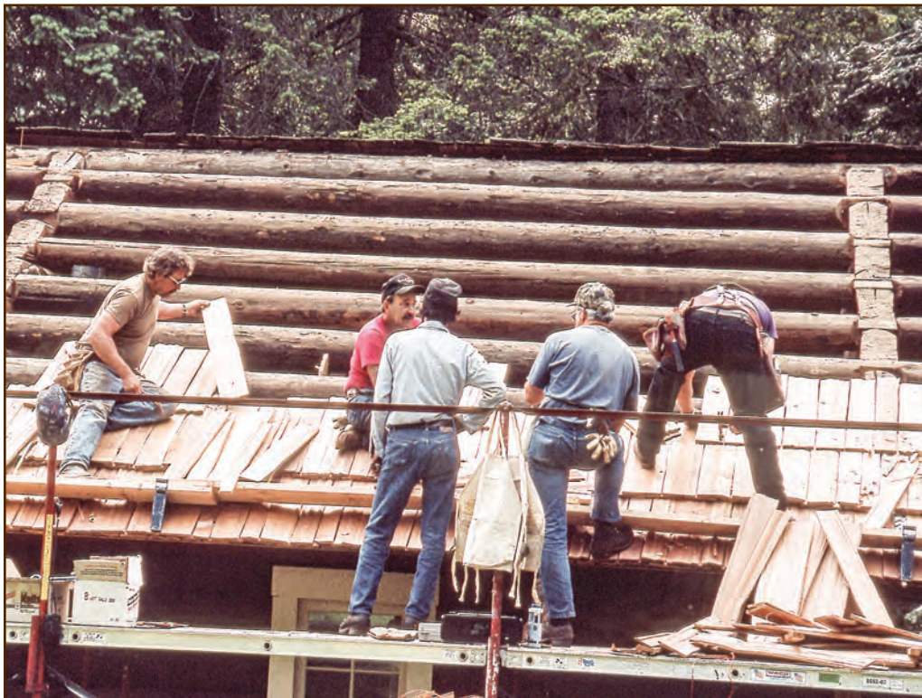
Figure 271—This crew laid 32-inch-long shakes on the purlin roof of the fire cache at the Moose Creek Wilderness Station (Nez Perce National Forest, Northern Region) during the 1990s. If they were laying the shakes today, they all would wear hard hats and would wear fall protection harnesses while working on the upper courses.
