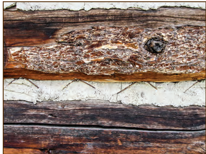
Figure E35—The builders tacked smooth wire to the logs in a zig-zag pattern to provide reinforcing for the daubing on the Fritz Cabin (Dubois Ranger District, Caribou-Targhee National Forest, Intermountain Region).
