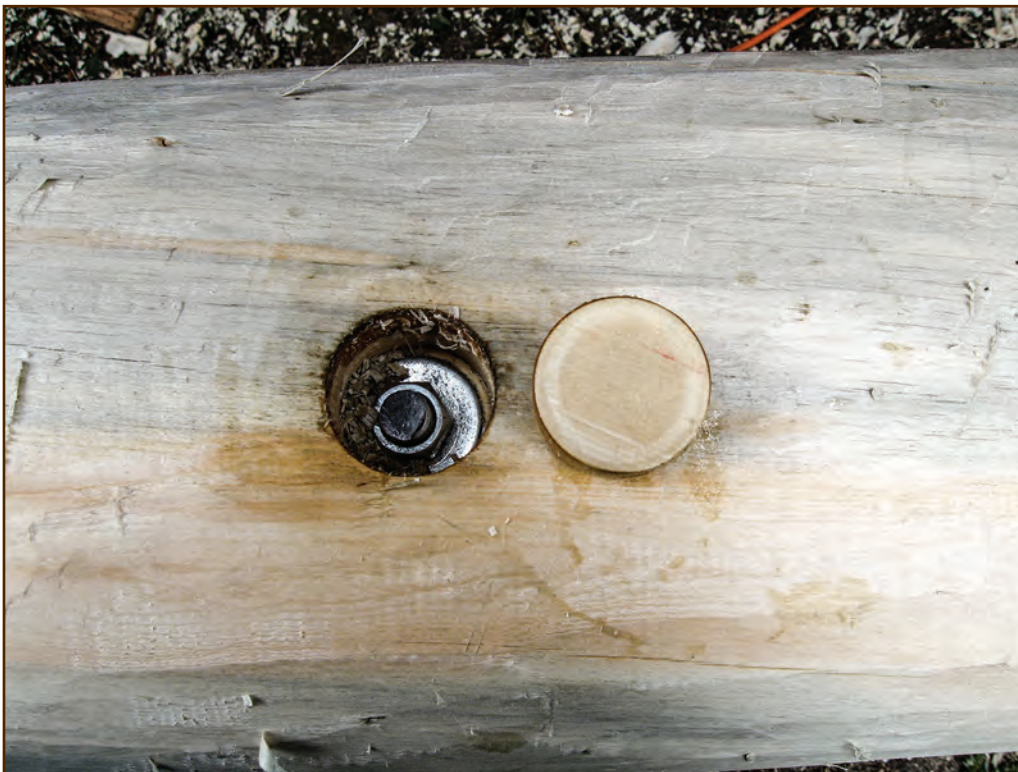
Figure 180—This closeup photo of the outside of a spliced log shows the recessed bolt, nut, and washer of a split-ring connector. The plug that the preservation crew will glue in place to cover the recessed bolt and nut sits on the log beside the recess.
