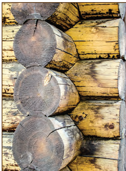
Figure E38—The builders coped the logs of this workshop, providing a tight fit between the logs. They used small wood inserts to more completely seal the space between logs at the crown ends, but daubing was not necessary. The workshop originally was a small barn built in 1936 on the Crandall Ranger Station (Shoshone National Forest, Rocky Mountain Region).
