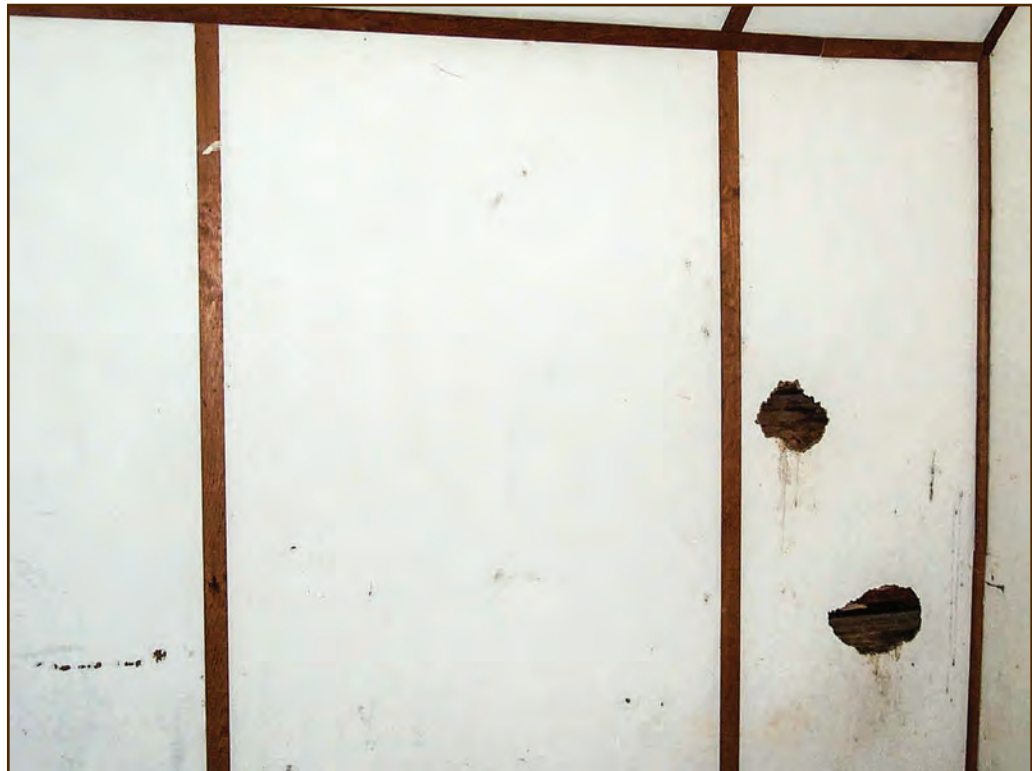
Figure 317—The original fiberboard covering the walls in the upstairs west bedroom at the Adams Ranger's House was damaged by water leaking through the roof, rodents, and vandalism.
