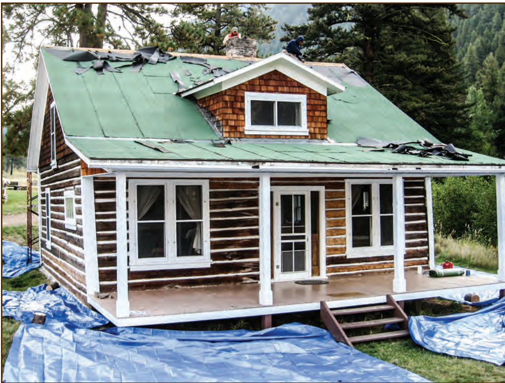
Figure 282—These roofers are replacing the old asphalt rolled roofing at Hogback Cabin (Lolo National Forest, Northern Region). The roofing had deteriorated along the unusual vertical seams. Roofers usually lay asphalt rolled roofing with horizontal seams.
