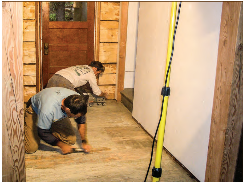
Figure 309—Preservation crewmembers patched, planed, and sanded the kitchen floor at the Adams Ranger’s House (Salmon River Ranger District, Nez Perce National Forest, Northern Region) before refinishing it.
