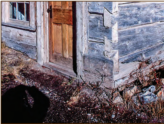
Figure E8—The builders constructed this cabin directly on the ground. The lowest logs of the cabin are rotting because the ground holds moisture against the logs, which enables fungi to invade the wood.
