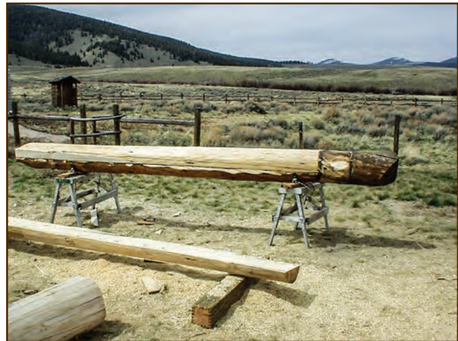
Figure 177—This photo shows a half-log splice in progress. The crew has not yet completely shaped the pale new wood to match the wood it will replace. This splice doesn't include the end of the existing log because the end was sound, and the crew didn't need to repair it. Using a half-log splice allowed the crew to keep the historic interior finish intact. It is always best to retain as much historic material as possible.
