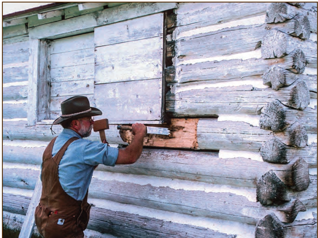
Figure 167—Preservation carpenter Bernie Weisgerber, now retired from the Forest Service Northern Region Historic Preservation Team, used a mallet and chisel to remove the deteriorated wood, which was more extensive than it appeared at the surface. Notice that he removed the chinking and daubing adjacent to the deteriorated area so that he could more easily access the damaged area.
