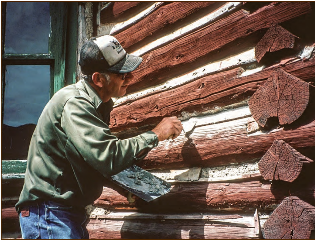
Figure 200—This preservation crewmember is using a small trowel to apply daubing to a cabin, carefully matching the profile of the new daubing to that of the original daubing. His hawk is nearly empty of daubing material.
