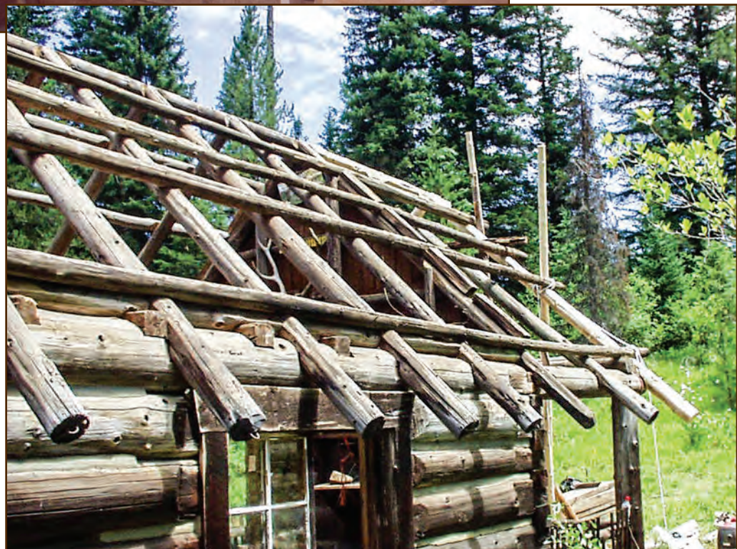
Figure 208—The Liz Creek Cabin (Clearwater National Forest, Northern Region) has a rafter and purlin roof structure. Because of decay, preservation crewmembers removed one of the purlins and the roofing, revealing the framing. They replaced these components before installing the new roofing.
