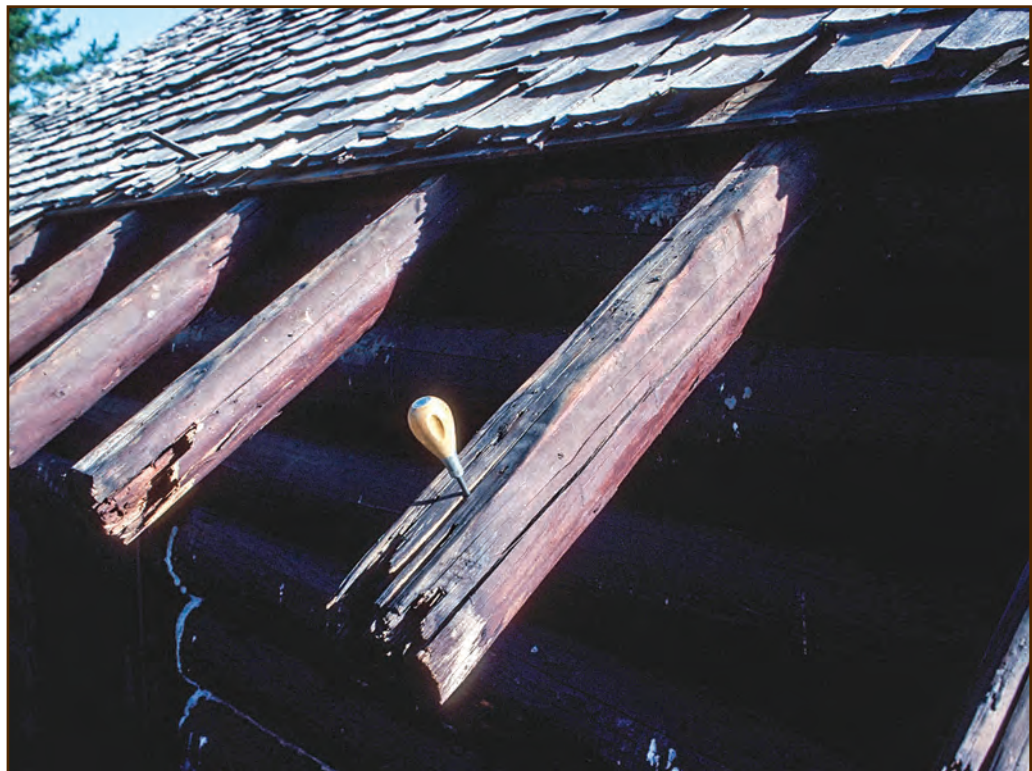
Figure 186—Preservation crewmembers removed the sheathing and roofing from these rotted rafter tails. The penetration of the awl into one of the rafter tails shows the depth of the rot. The crew will have to remove about a foot from the ends of these rafters.
