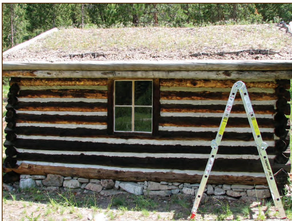
Figure 289—When preservation crewmembers replaced the sod roof of the Alta Ranger Station, they put down a layer of ethylene propylene diene terpolymer (EPDM) over the puncheon sheathing, then laid geocell to hold the soil in place. Unfortunately, the crew had to remove the geocell fabric after it warped and emerged from the soil.
