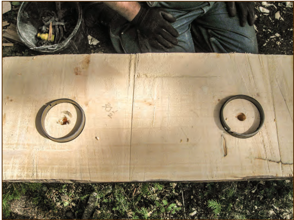
Figure 179—Preservation crewmembers recessed split-ring connectors halfway into this splice. They also will recess the connectors halfway into the old log. Next, they will put the splice and log together, thread the bolt through the matching center holes in the splice and old log, and secure the connection with nuts and washers.
