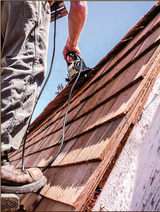
Figure 264—This roofer is using a small circular saw to cut off the first course of shingles on the gambrel of the stud barn at the Nine Mile Ranger Station (Lolo National Forest, Northern Region).
