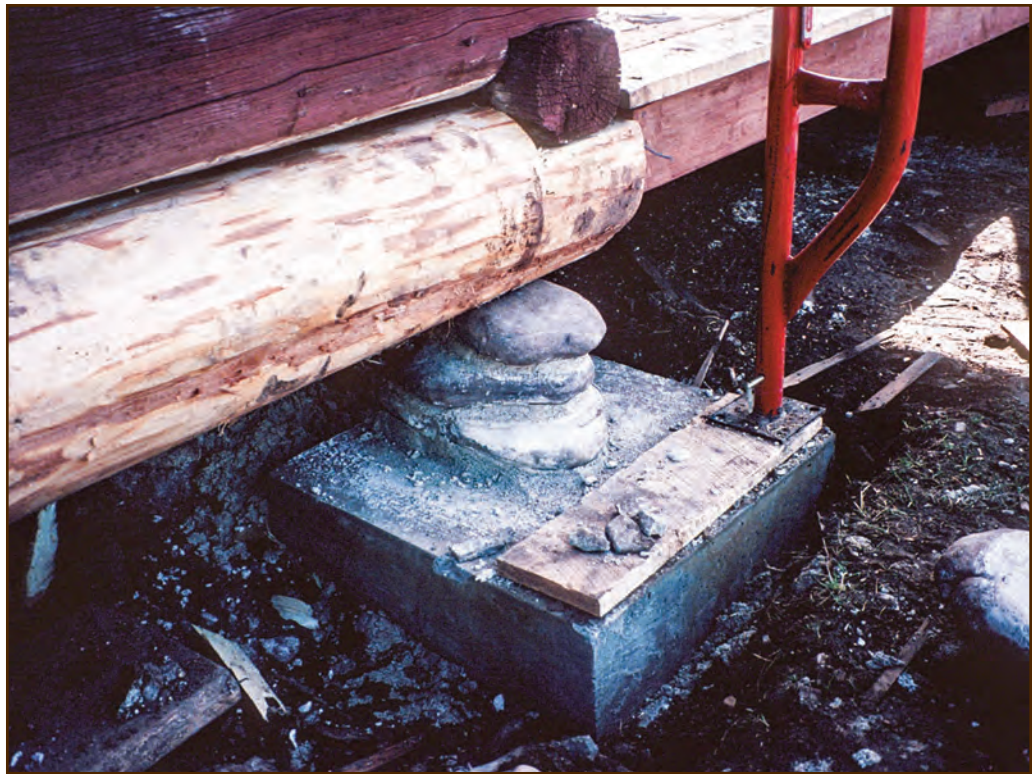
Figure 81—Preservation crewmembers constructed a new footing and stone pier at the Judith Guard Station of the Lewis and Clark National Forest, Northern Region. The footing is under a corner of the cabin where the wall meets the porch.
