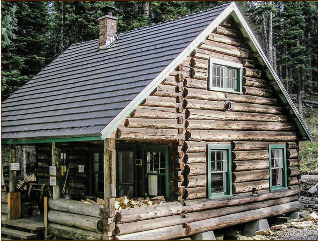
Figure 307—The original brick chimney at the Adams Ranger’s House (Salmon River Ranger District, Nez Perce National Forest, Northern Region) had deteriorated so badly that preservation crewmembers had to completely rebuild it. Although the crew replaced the portion of the chimney inside the building (hidden inside the interior walls) with a lined concrete block chimney, they rebuilt the portion visible above the roof to the original proportions using the original bricks.
