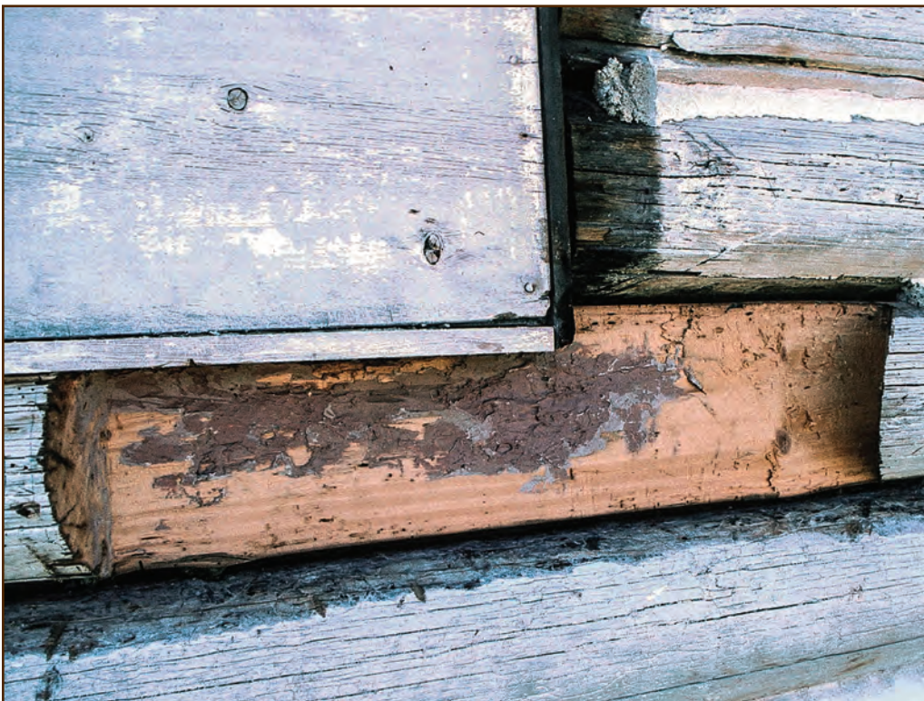
Figure 169—There is a small epoxy patch at the back of the finished cut out area. The log is dry and the epoxy and surrounding wood will be well protected from moisture in this location once the preservation carpenter replaces the chinking and daubing.
