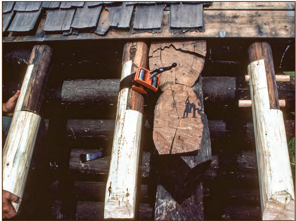
Figure 190—This photo shows three stages of rafter tail replacement using a lap joint. On the left, a preservation crewmember checks the fit of the replacement rafter tail. In the middle, the crewmember applied epoxy adhesive to the cut faces of the existing log and clamped the replacement rafter tail in place. On the right, he inserted the glued dowels into the drilled holes.
