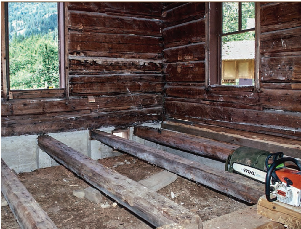
Figure 132—The builders set the floor joists at the Bull River Guard Station (Kootenai National Forest, Northern Region) on piers cast with the concrete foundation when they constructed the building in 1907. Over time, the foundation failed. Preservation crewmembers reinstalled the original floor joists on piers cast with the new foundation that exactly matched the original piers.
