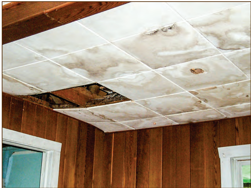
Figure 53—The original fiberboard ceiling tiles shown in this photo (taken before renovation of the living room at the Adams Camp Ranger’s House) are moldy and damaged by moisture.
