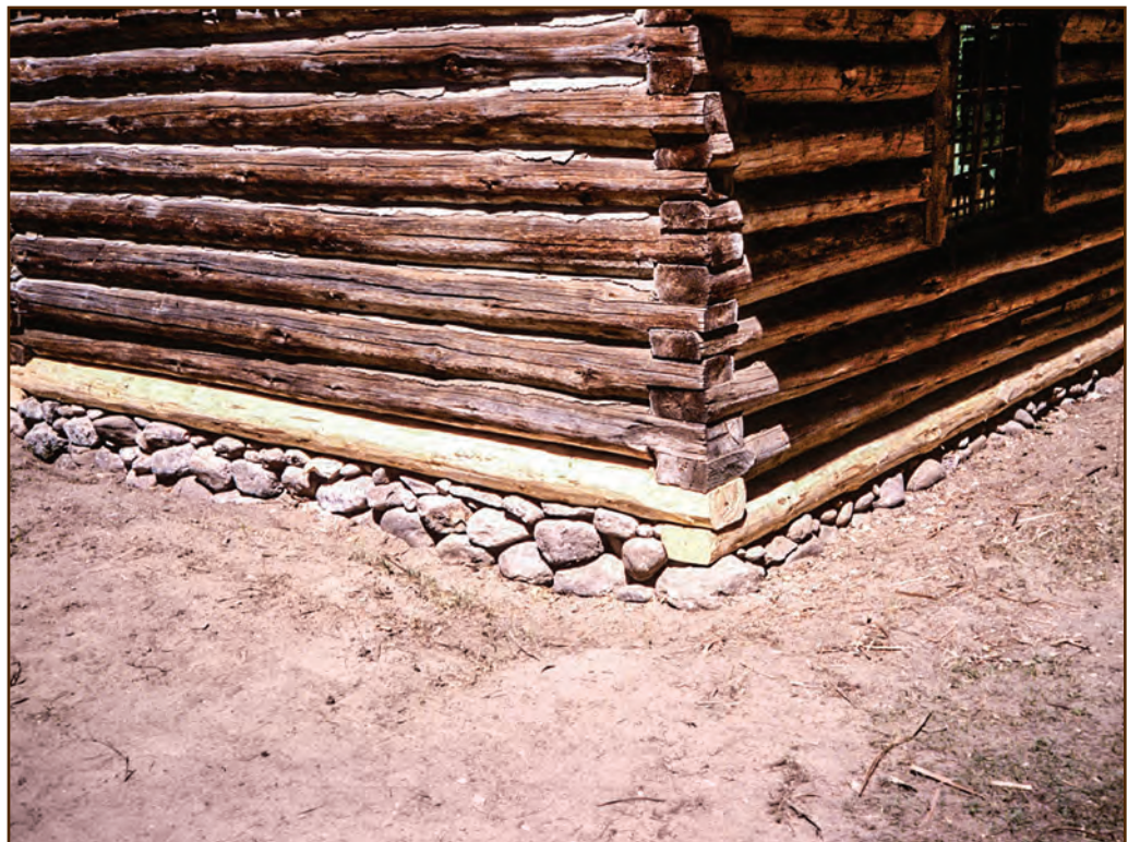
Figure 87—Preservation crewmembers constructed a new cobblestone foundation under the Cooper's Flat Cabin in the Bitterroot National Forest, Northern Region.
