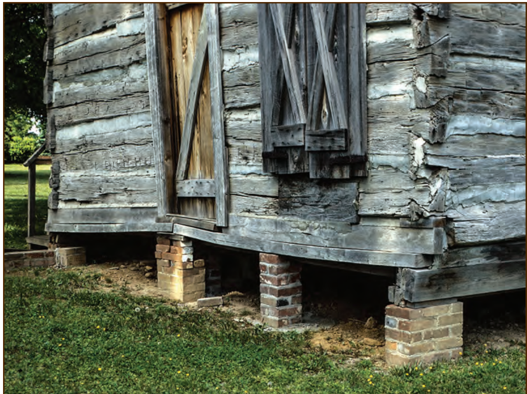
Figure 46—This building shows evidence of several inappropriate “repairs.” The piers supporting the building are of different types of brick and were constructed using at least three different construction methods. Someone used modern dimensioned lumber to replace the sill and spandrel logs. The door may originally have been located where a log “patch” is placed under what is now a shuttered window. People used at least two different styles and materials for the daubing. Someone also used daubing material to “patch” deteriorated areas on the ends of some of the logs.
