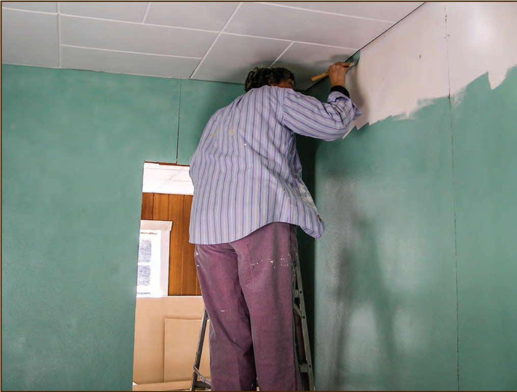
Figure 292—Preservation crewmembers repainted the original seafoam green color on the fiberboard bathroom walls they repaired at the 1933 Adams Ranger’s House (Nez Perce National Forest, Northern Region).
