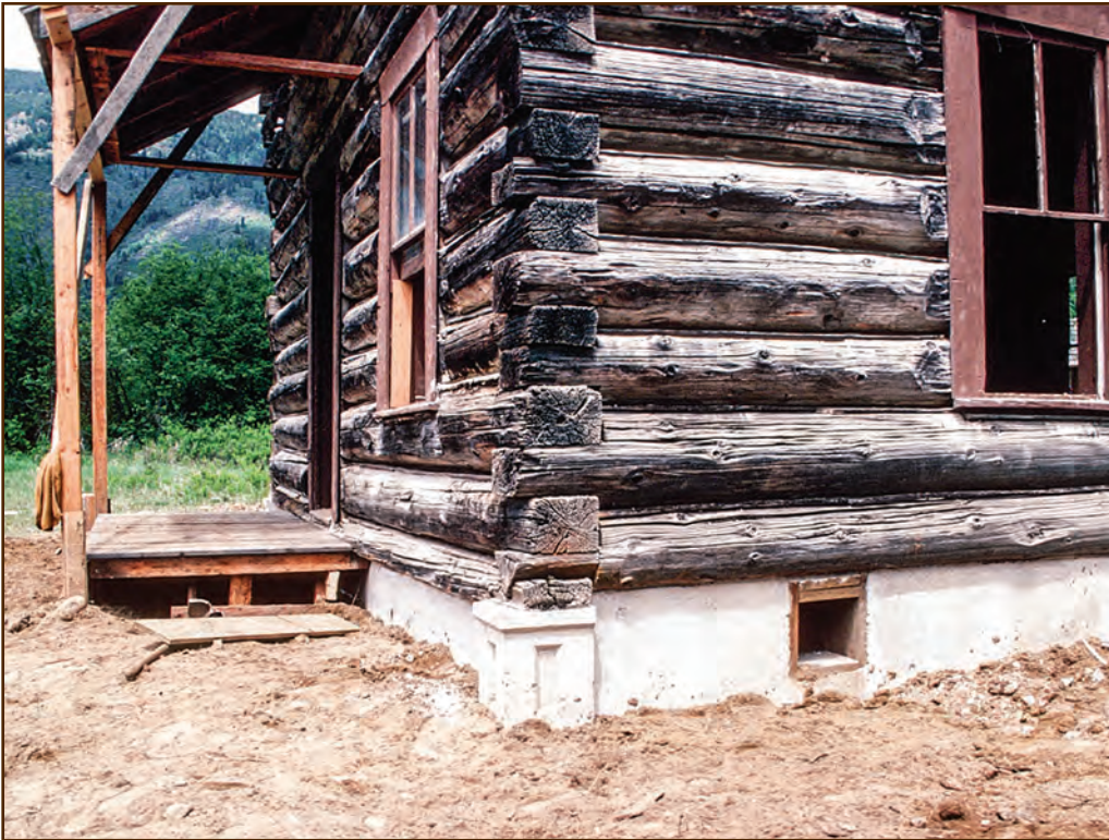
Figure 86—The completed replacement foundation matches the appearance of the original foundation, including the forming details on the corners. Preservation crewmembers created foundation vents out of the gaps in the foundation through which the steel beam needles extended.
