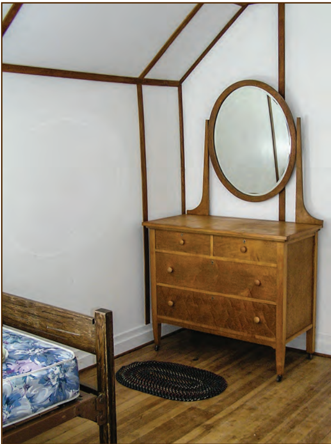
Figure 319—The preservation crew replaced damaged sections of fiberboard in the west bedroom with similar modern fiberboard panels, reinstalled the original wood battens to cover the panel joints, and replaced or reinstalled the trim boards. The crew painted the panels, battens, and trim boards to match the original colors.
