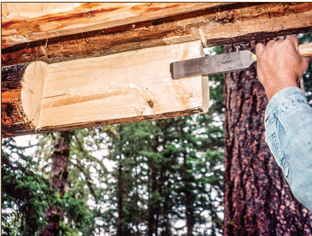
Figure 188—A preservation crewmember used a saw to cut the shape for a half lap joint on this purlin end, and a chisel to smooth the face flat.
