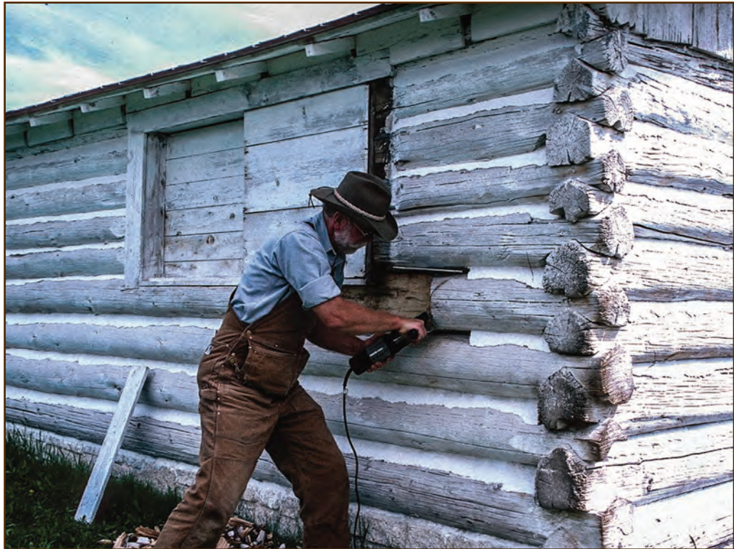
Figure 168—The preservation carpenter used a reciprocating saw to cut a clean edge at an angle on the end of the cut out area.
