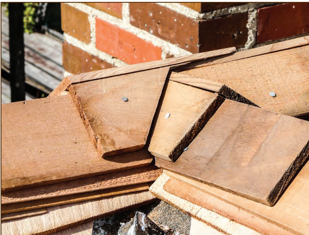
Figure 276—Preservation crewmembers constructed this complex shingle ridge cap while replacing roofing on the Zortman Guard Station within the Bureau of Land Management’s HiLine District in Montana. The shingle butts switch direction in the middle of the roof peak, and a cross gable also intersects the main ridge line at that point. Because of the cross gable, the crew cut a notch into one side of the ridge cap unit at the middle of the roof.
