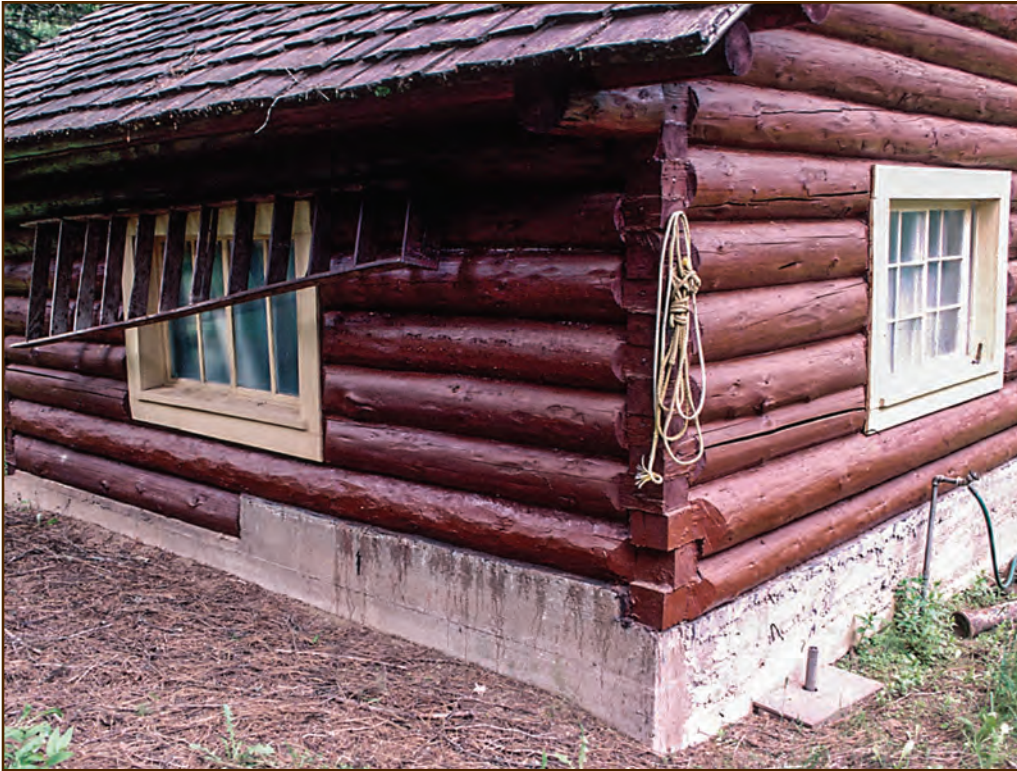
Figure 37—When some of the lower logs of this building rotted out, someone added a concrete wall to replace the sill logs, spandrel logs, and some wall logs; added a concrete foundation; and replaced some of the wall logs with new logs. One of the new logs was roughly debarked, making it look different from the older logs. Concrete is not an appropriate “repair” for rotted logs.
