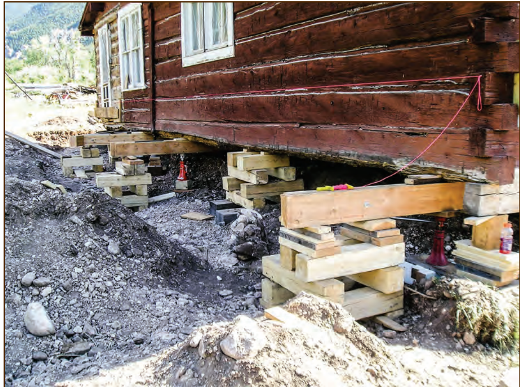
Figure 72—Preservation carpenters stacked cribbing in several locations under needles and solid logs to support the Sage Creek Cabin (Custer National Forest, Northern Region) as they raised the cabin using jacks.
