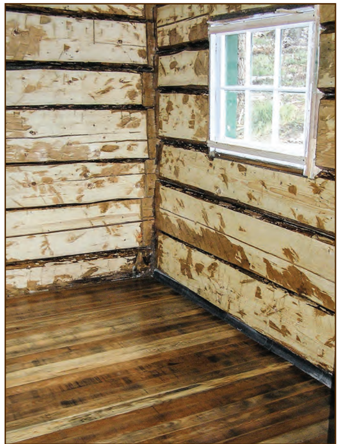
Figure 314—The builders hewed and rough sanded the insides of the log perimeter walls at the kitchen and bathroom of the Adams Ranger's House to form a relatively flat surface. The builders originally covered the logs with fiberboard, but the fiberboard was severely deteriorated and the preservation crew did not replace it in the kitchen or bathroom when they repaired the cabin.
