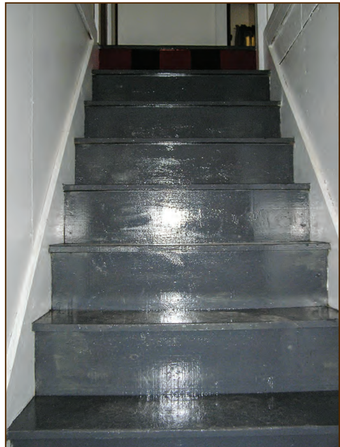
Figure 313—Preservation crewmembers painted the repaired stairs in the Adams Ranger's House glossy gray to match the original finish.
