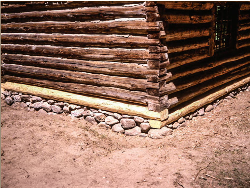
Figure 151—Preservation crewmembers replaced the sill and spandrel logs, and this cabin once again sits on its foundation rather than on cribbing and jacking.
