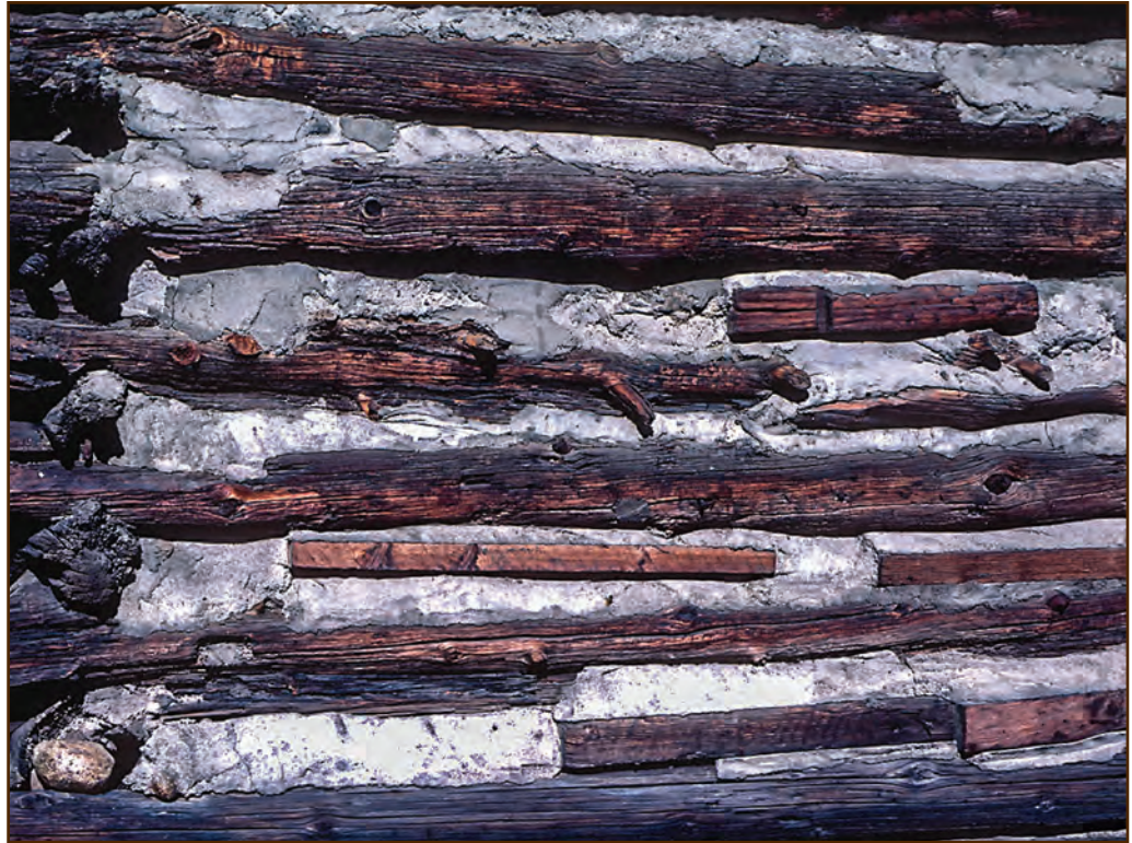
Figure 35—Someone “repaired” the daubing on this cabin with a concrete mortar mix and an odd use of wood scraps. The “repairs” don’t match the original materials or methods and probably are contributing to further decay of the logs.
