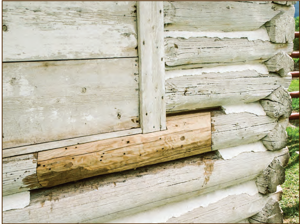
Figure 172—The ends of the angled dowels are darker ovals that are visible toward the ends of the splice. The epoxy has cured and the preservation carpenter has removed the band clamp.
