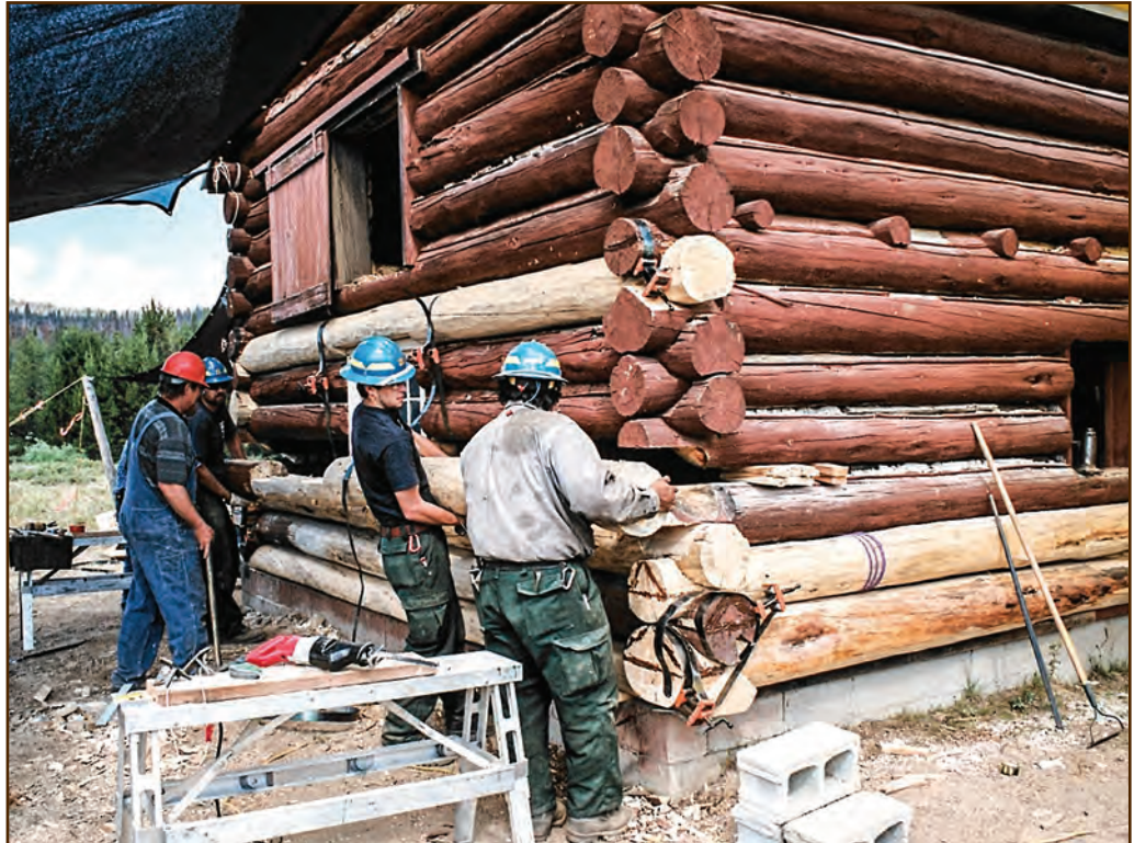
Figure 138—This preservation crew is lifting a replacement log into position at the Landmark Ranger Station barn of the Intermountain Region’s Boise National Forest. One crewmember holds the shaft of a large mallet that he will use to knock the log into its final position.
