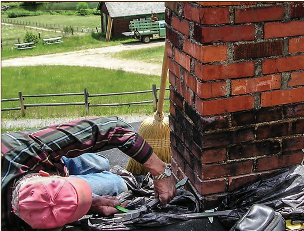
Figure 243—This preservation crewmember is using a hammer and plugging chisel to rake the joints on the chimney of a house built in 1905 at the Main Boulder Station (Gallatin National Forest, Northern Region).
