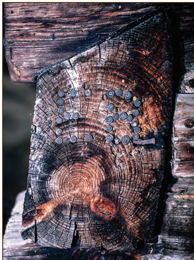
Figure 34—The initials “EB” (most likely for Ernest Betasso), made by hammering bullet casings into the end of a log, are an example of a detail that should be recorded in a historic assessment. This interesting feature was found at the Betasso Ranch Preserve “homestead cabin” near Boulder, CO.
