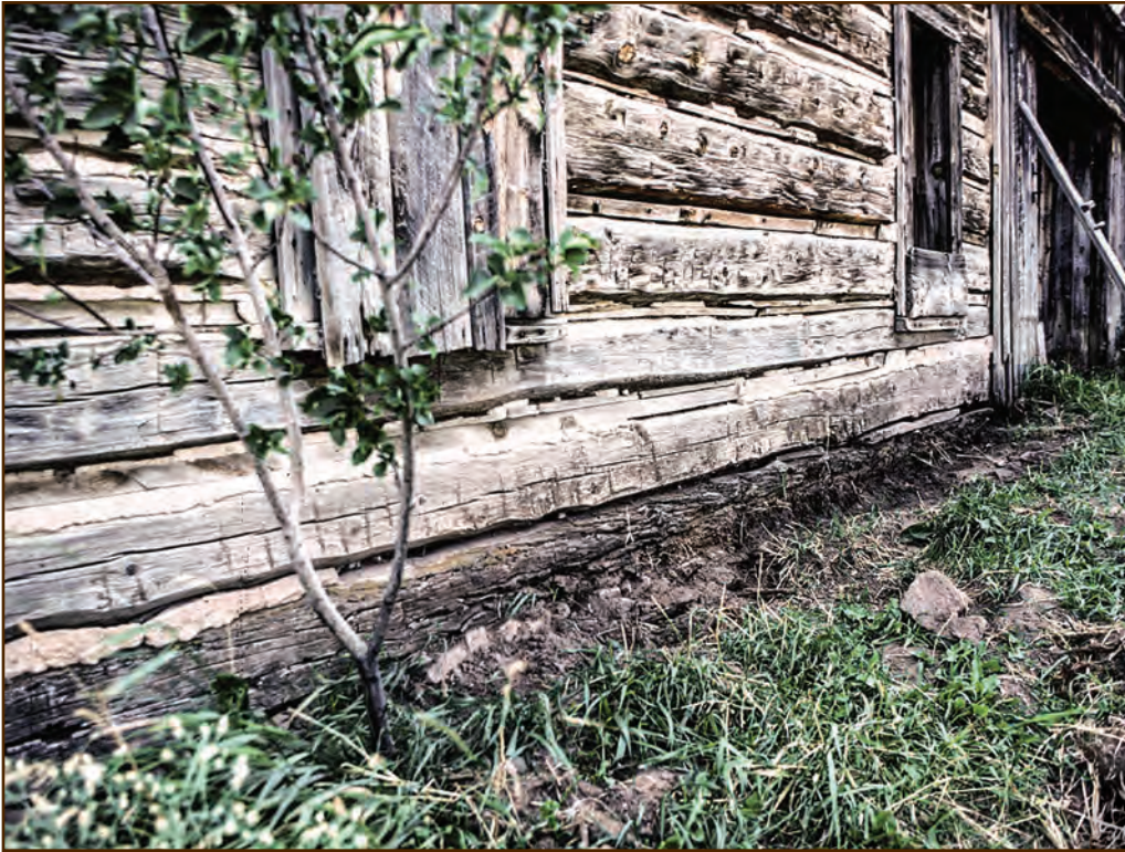
Figure 42—Constant contact with the ground has seriously decayed the sill log of this building.
