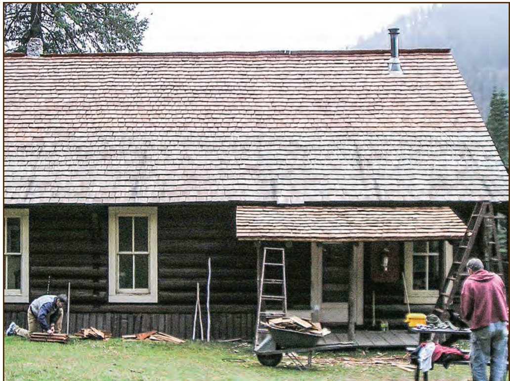
Figure 224—The cock's comb ridge cap is clearly visible on the skyline of the newly reroofed Office/Cookhouse building at the Moose Creek Wilderness Station (Nez Perce National Forest, Northern Region).
