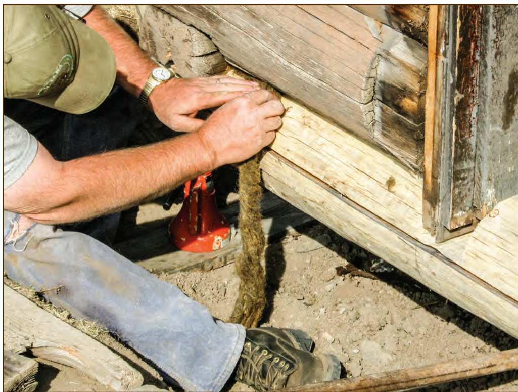
Figure 199—This preservation crewmember is stuffing oakum chinking into the gaps between the logs at the Gates Park Guard Station cabin (Lewis and Clark National Forest, Northern Region). After filling the gaps, he will apply the daubing.
