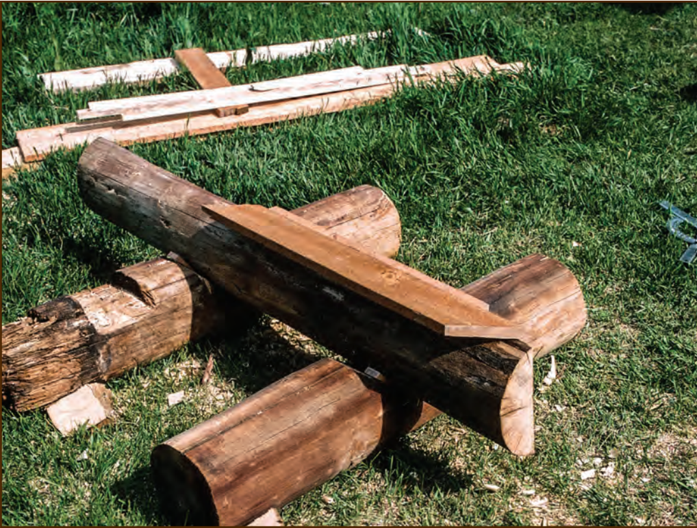
Figure 170—The preservation carpenter cut a board to match the length and angles of the cut out area as a pattern for cutting the splice.
