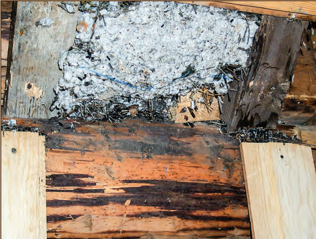
Figure 54—The renovators uncovered this rodent nest studded with droppings when they removed damaged fiberboard wall and ceiling panels at the Adams Camp Ranger’s House.
