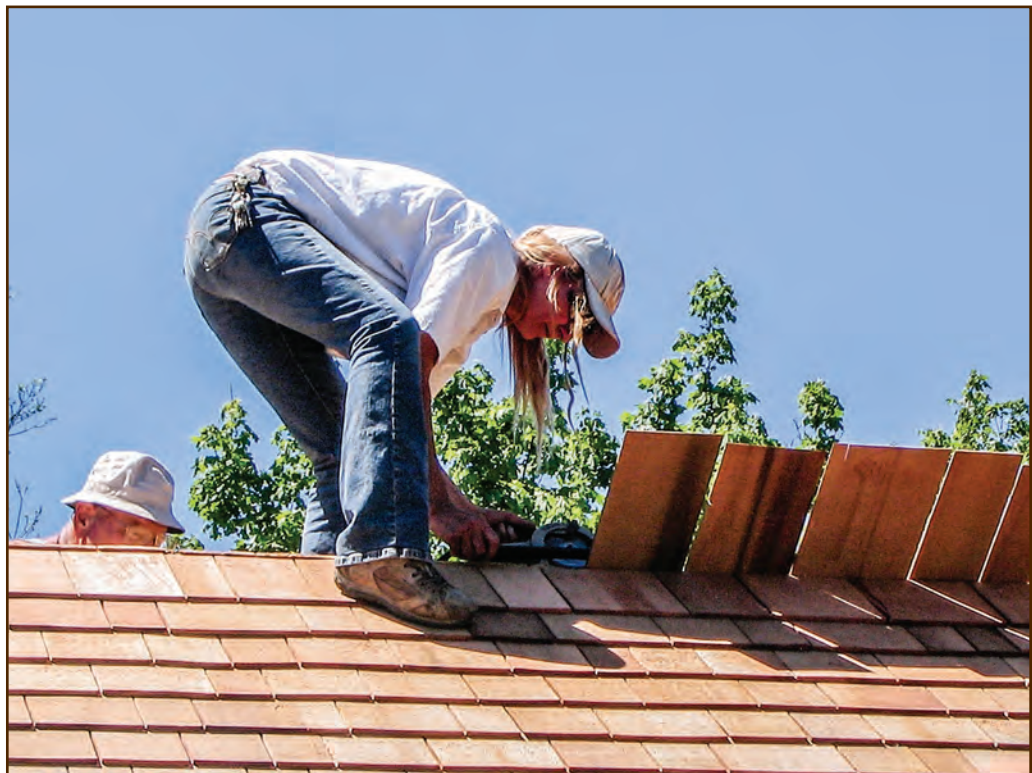
Figure 267—This roofer is using a small circular saw to cut the tails off shingles near the ridge of a roof.
