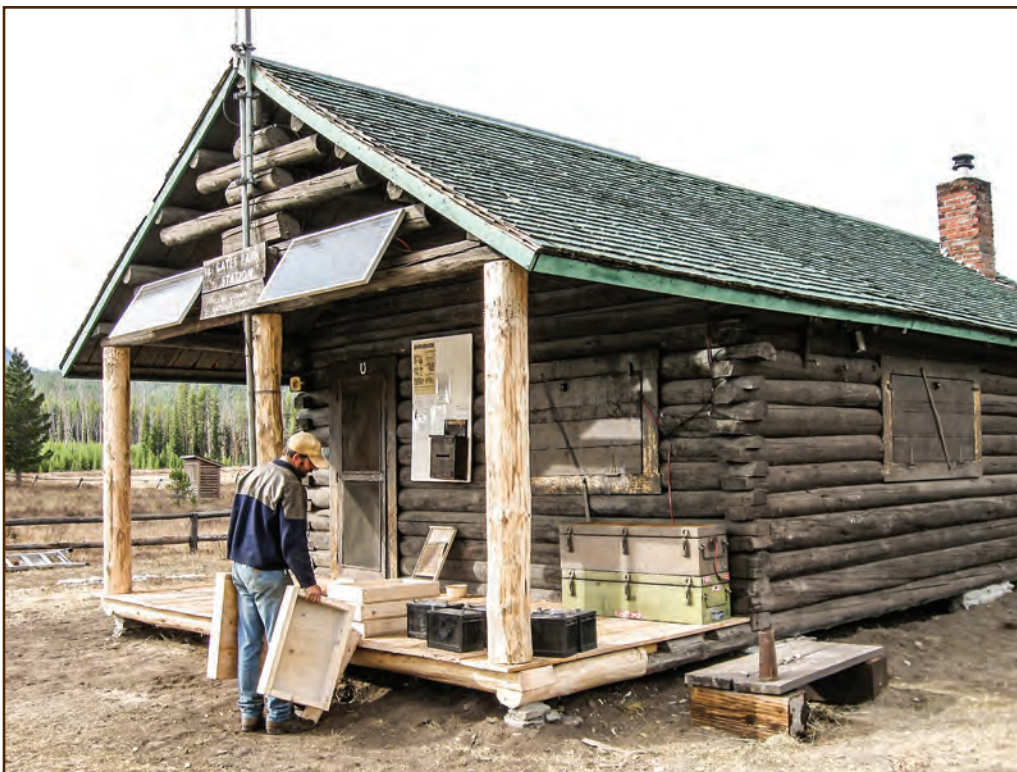
Figure 176—Preservation crewmembers replaced the ends of the porch sill logs at the Gates Park Station cabin (Lewis and Clark National Forest, Northern Region) using end-to-end log splices. They replaced the porch foundation, spandrel log, posts, and floor boards at the same time.
