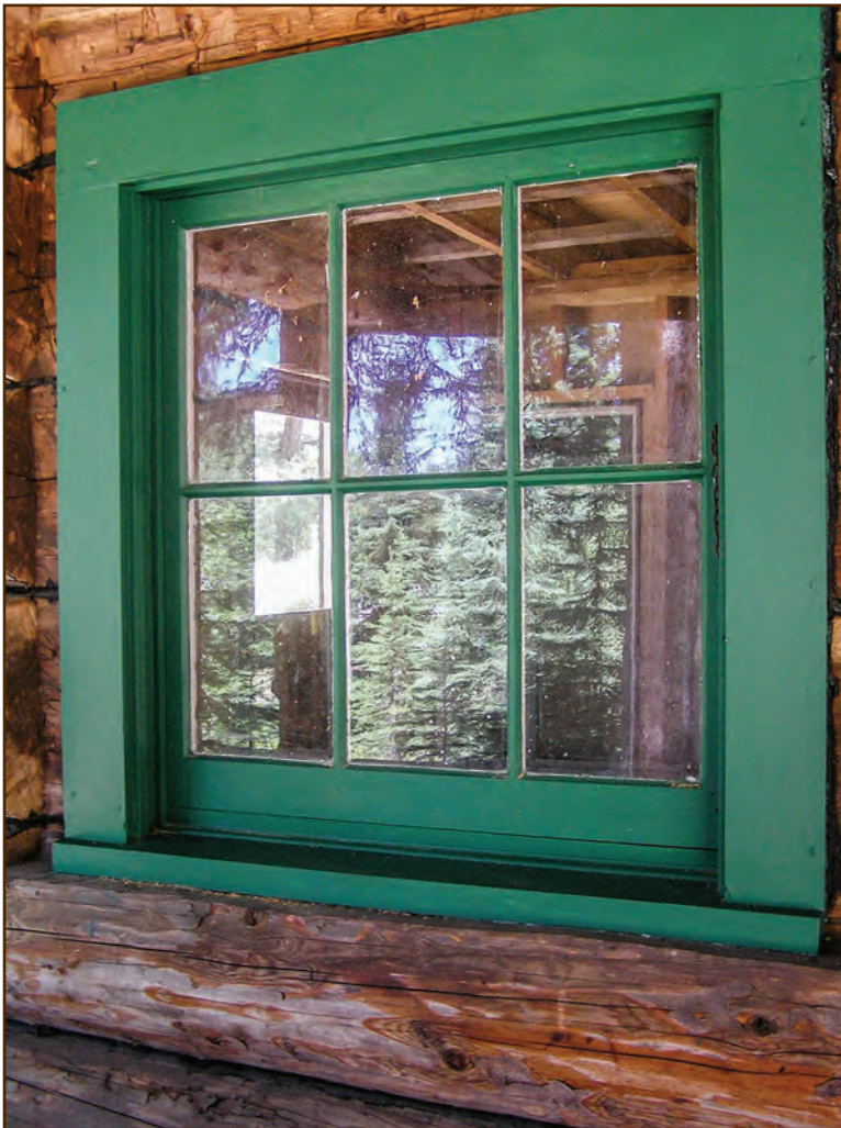
Figure 301—As part of the restoration work at the Adams Camp Ranger’s House on the Salmon River Ranger District (Nez Perce National Forest, Northern Region), preservation crewmembers rebuilt this kitchen window and painted it a deep green to match the original paint. This particular green was a standard color in the Northern Region when the builders originally constructed the cabin in 1933.
