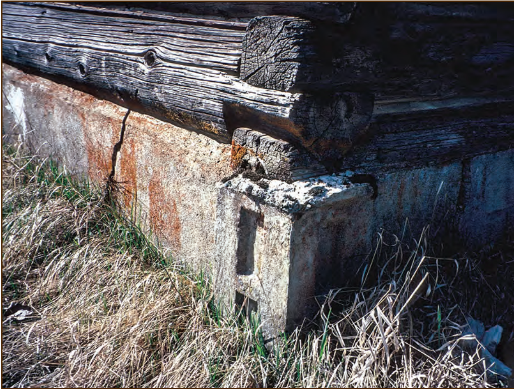
Figure 83—This foundation corner is cracked and leans out, but it's more intact than the rest of the foundation under the Bull River Guard Station of the Kootenai National Forest, Northern Region. The forming details in the concrete are important to the appearance of the building.
