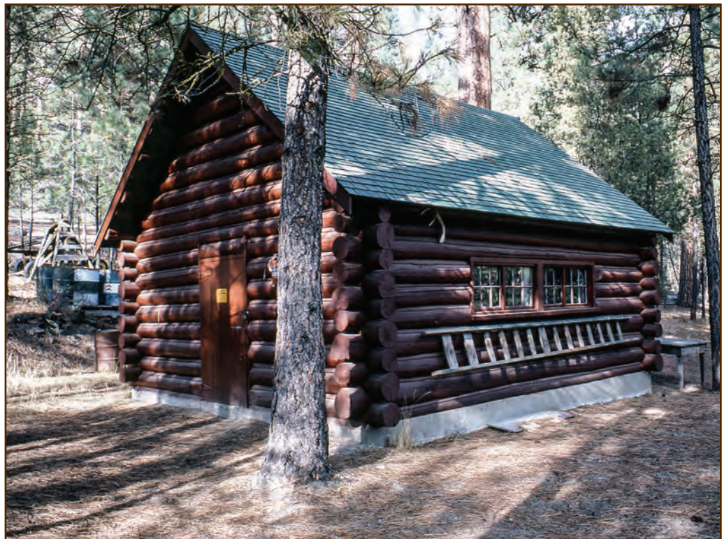
Figure 40—The ground should always slope away from the building, as shown in this photo of the 1931 Indian Creek Warehouse/Shop, so that runoff water is directed away from the structure. The building was moved from the Salmon River Guard Station to the Indian Creek Guard Station (both in the Boise National Forest of the Intermountain Region) in 1968.
