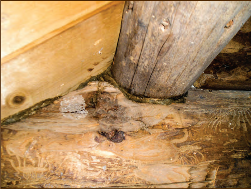
Figure 193—Preservation carpenters stuffed oakum into all the spaces between logs in the attic at the Moose Creek Wilderness Station Office/ Cookhouse building to keep bats out. Before crewmembers filled the voids and replaced the roof with shakes over continuous sheathing, several hundred bats occupied the attic each summer, creating an undesirable guano mess.
