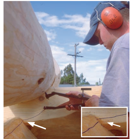
Figure 3: The groove was scribed, then the scribes were closed down slightly, and now Olaf is scribing the notch. The notch scribe line is a little above the groove scribe line—the difference in height is the underscribe amount.
