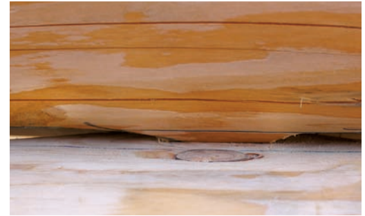
Figure 7.d: Close-up of a tab on a one-notch log. The purpose of the tab (or a wedge) is to keep the long groove's underscribe gap open. Here you can see the gap to the left and right of the tab. Over time, the tab crushes, and the underscribe gap will decrease towards zero. If needed, you can reach in with a saw, and cut the tab shorter to keep the gap in the groove equal along each log's length.
